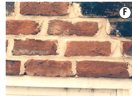
MASONRY IN POOR CONDITION
