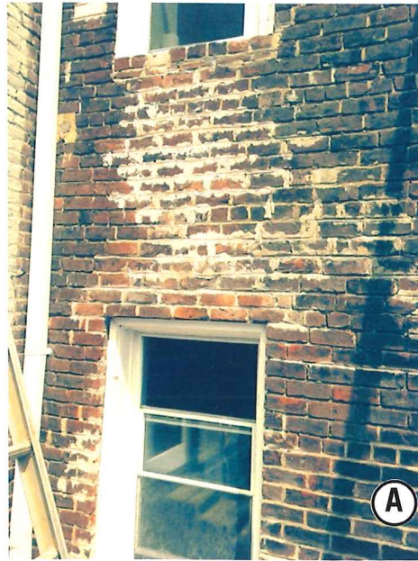
MASONRY IN POOR CONDITION
