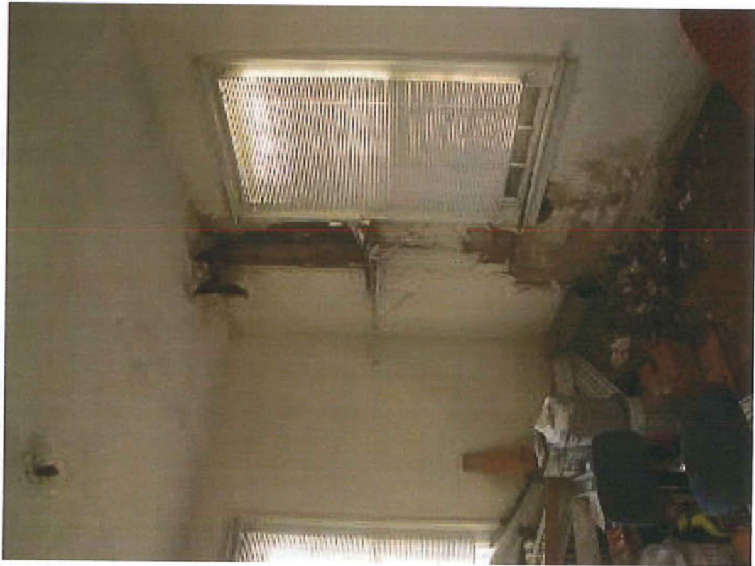
“South” Bedroom and damage
