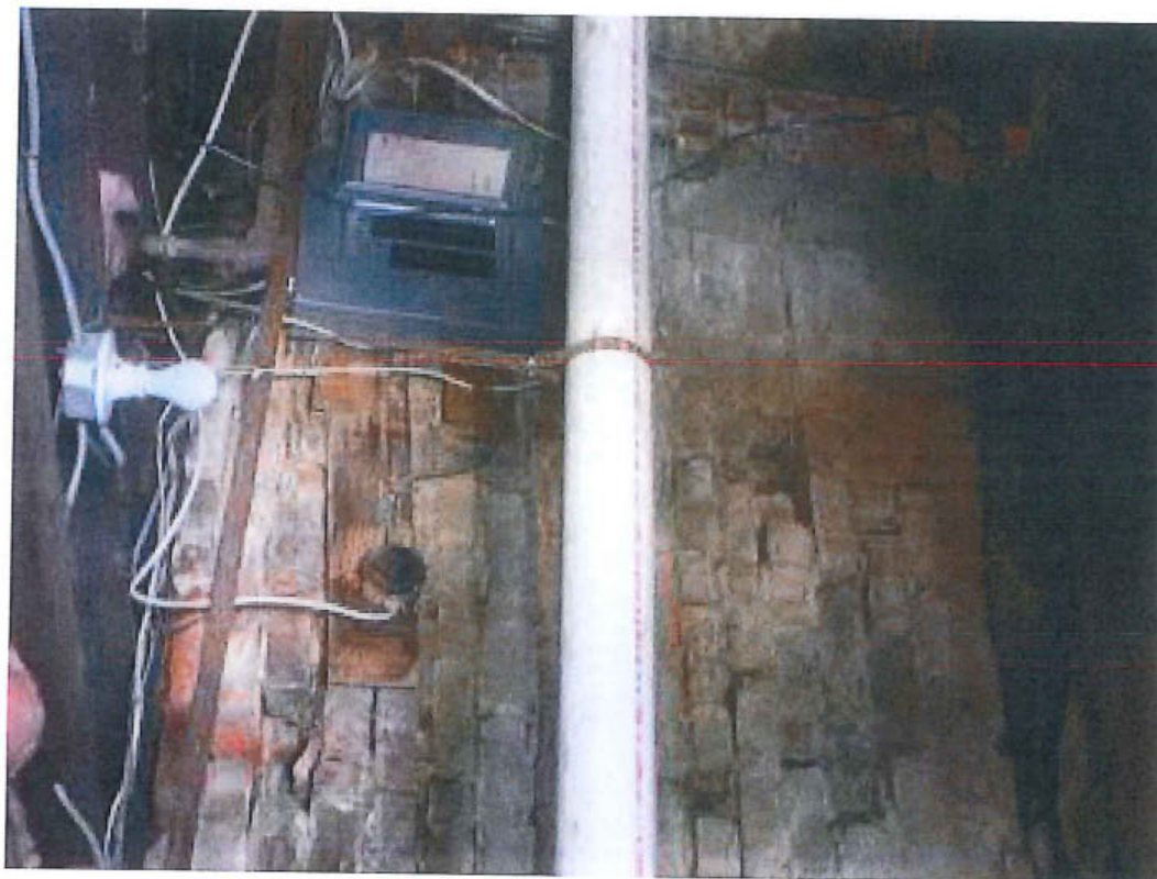
Electric Panel and West Foundation Wall
