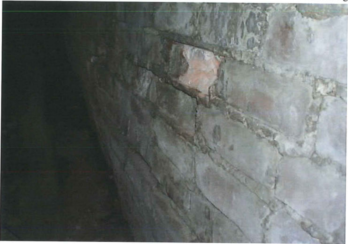
Bulging Foundation Wall at Street Side
