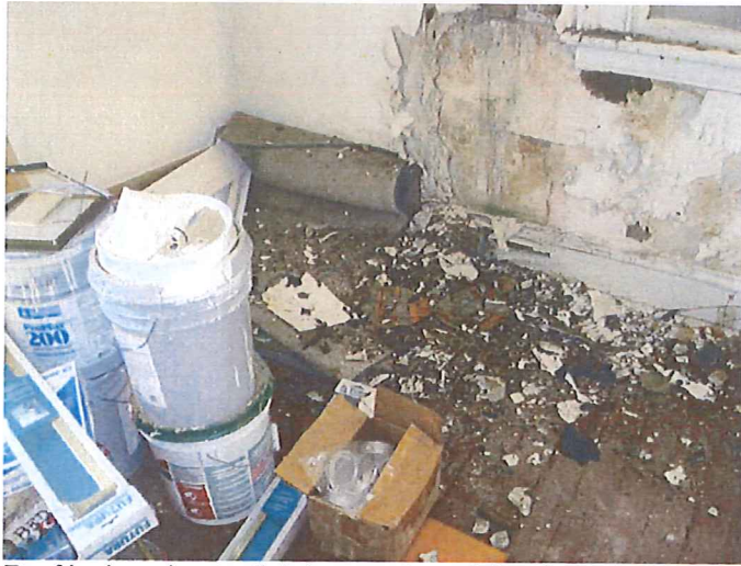
Roof leak and potential damage to wall framing.
