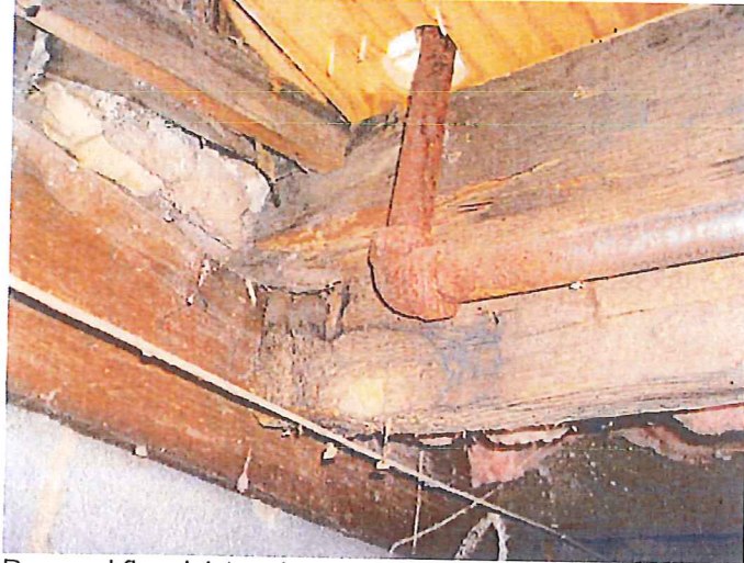
Decayed floor joist end
