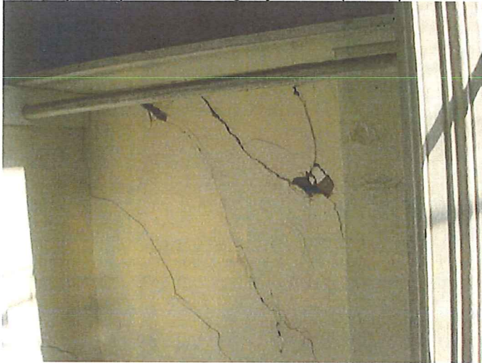
Cracked plaster at interior partition wall
