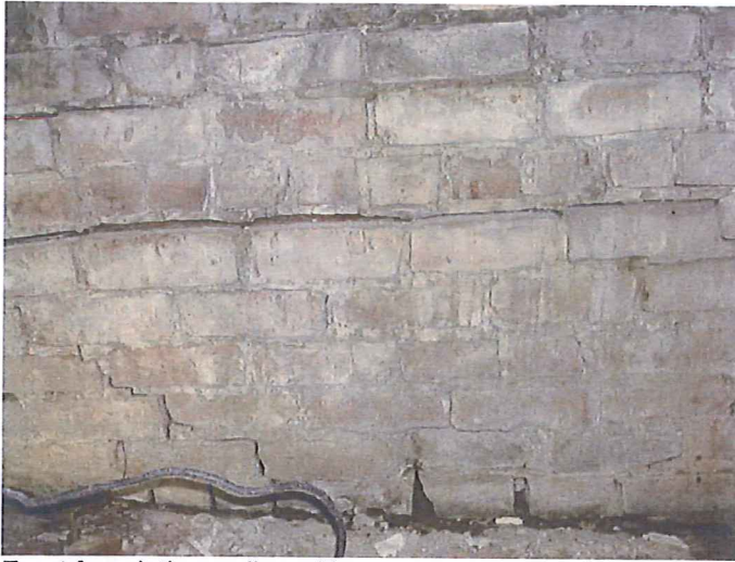
Front foundation wall cracking
