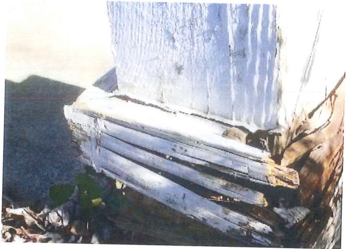
Deteriorated Post Base
