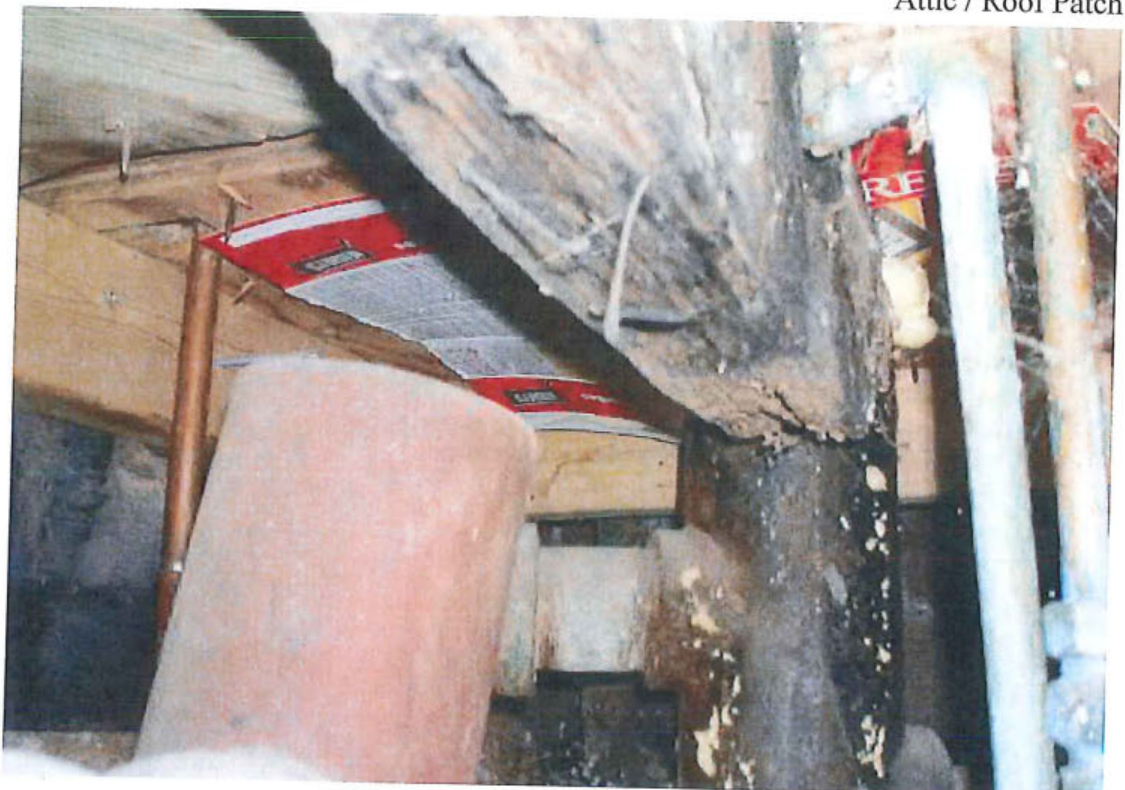
Primitive Floor Patch / Rotten Beam
