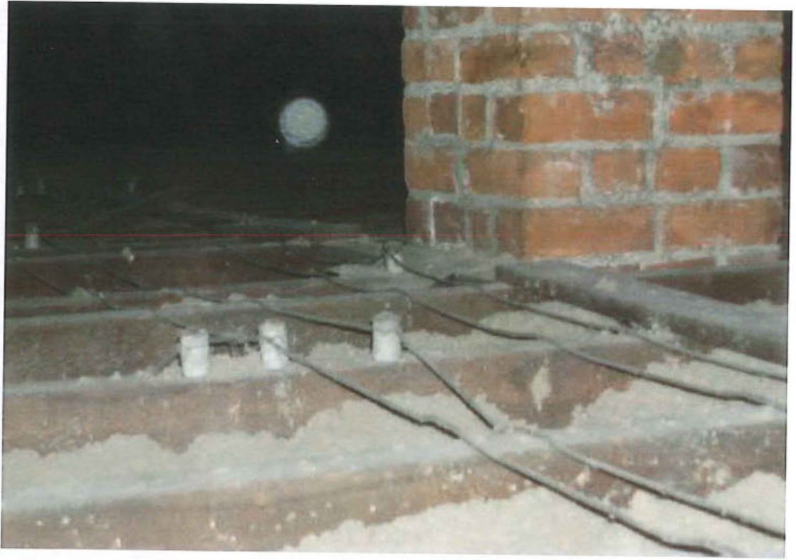
“Knob and Tube” Wiring in Attic
