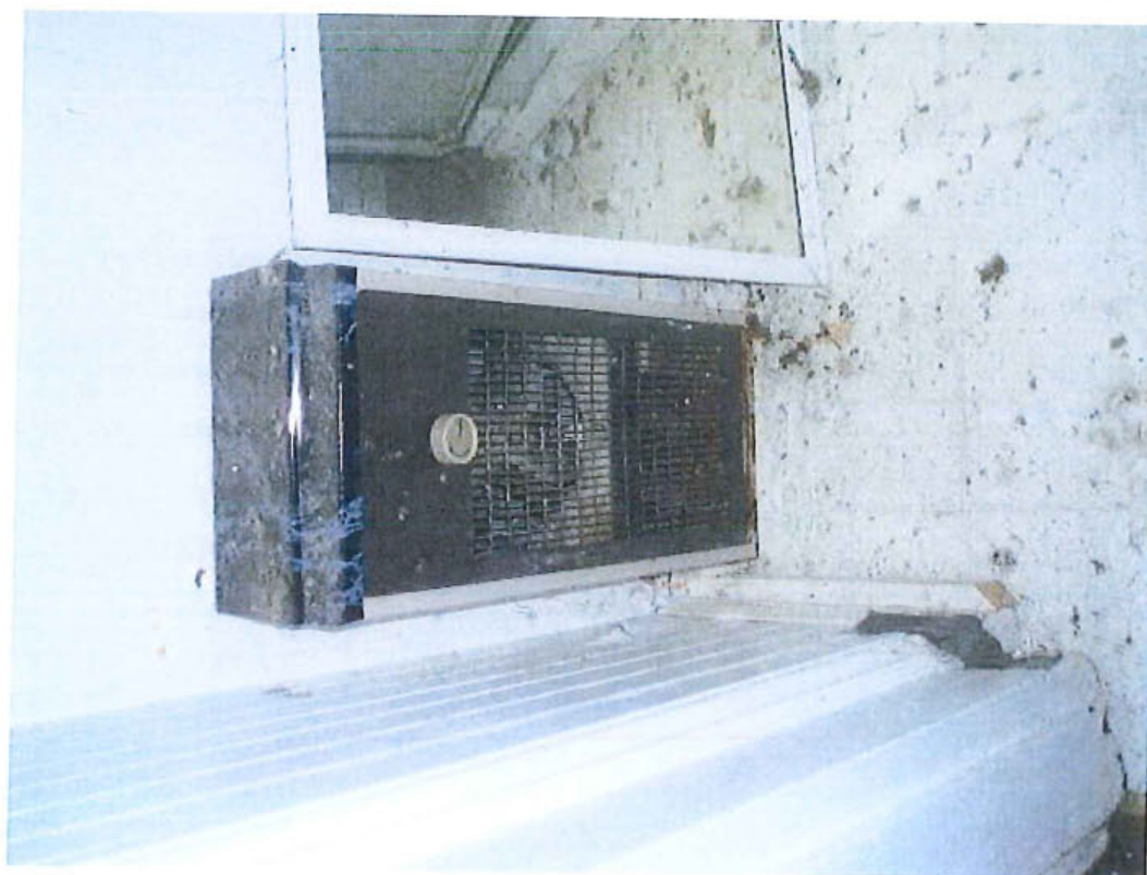
Electric Heater in Bathroom
