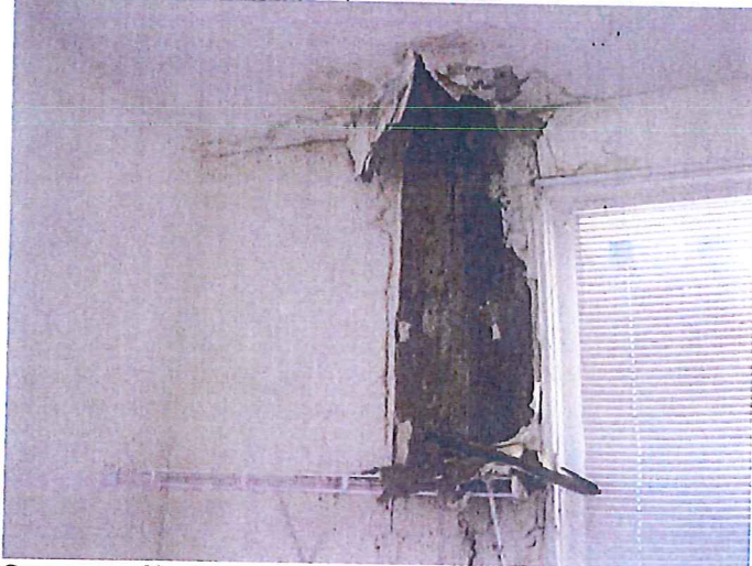
Severe roof leak
