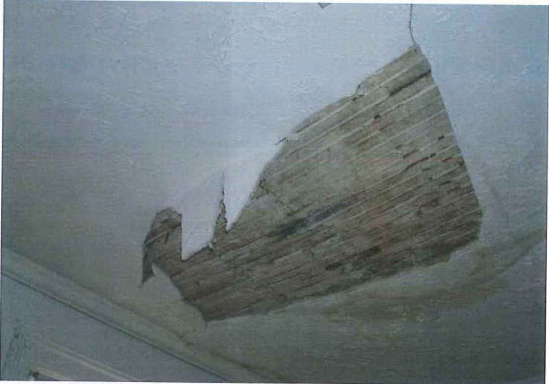
Roof Leak / Ceiling Failure
