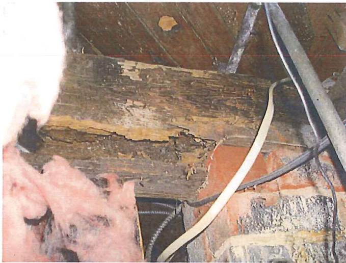
Severely decayed and damaged joist end (below partition wall)
