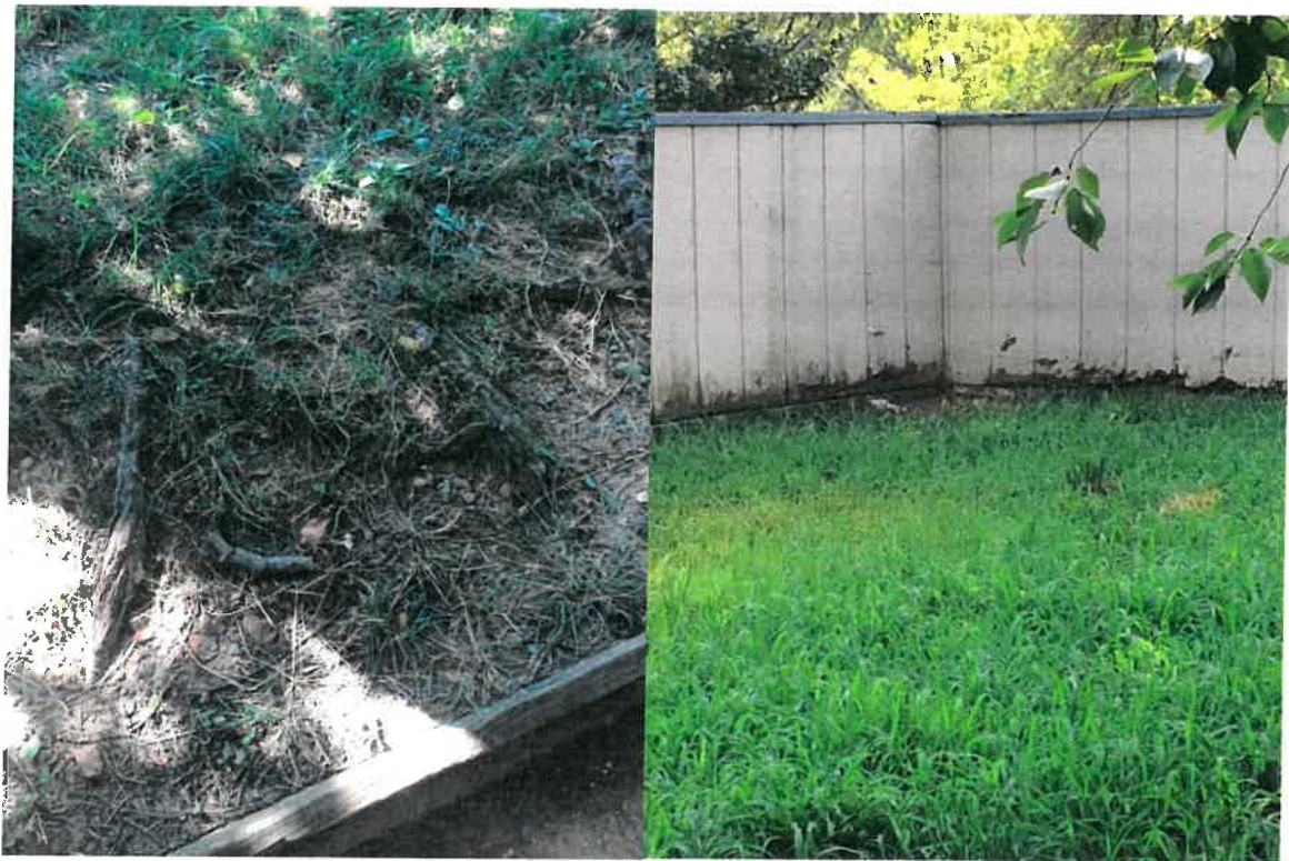
Moisture damage, rotting structures, encroaching root damage
