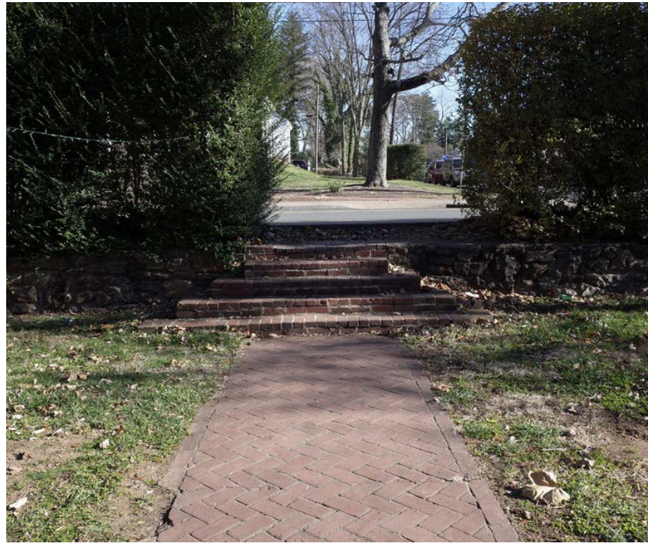
BRICK PAVERS, ENTRY STAIR, AND SITE WALL IMAGE TAKEN FROM ADJACENT PROPERTY (513 RUGBY ROAD)
