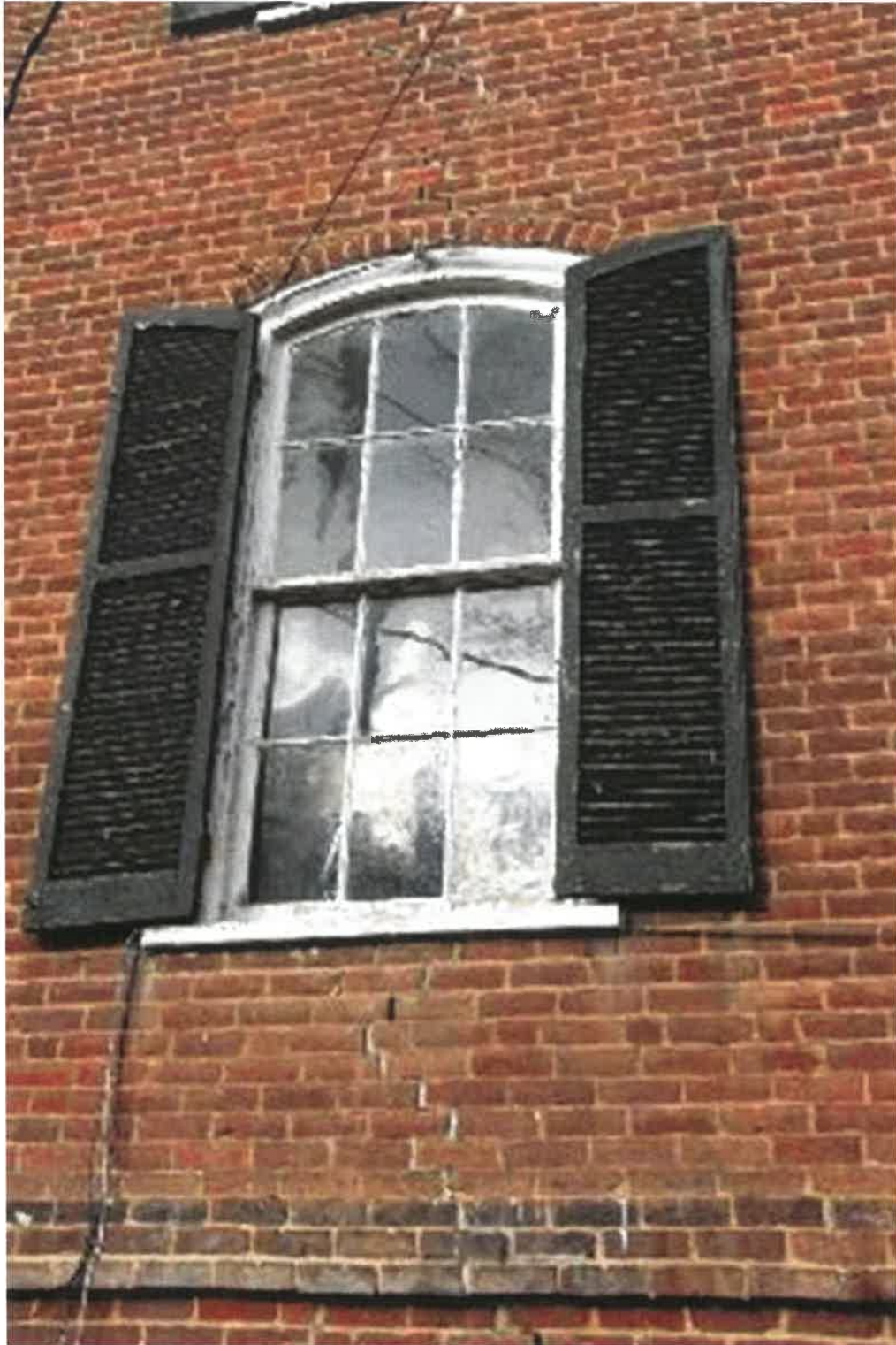
Typical Exterior Wood and Paint Conditions, and vertical masonry cracks
