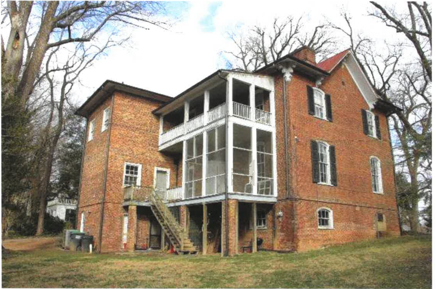
1920s Porch with recent pressure-treated stairs and 'temporary' supplemental structural posts
