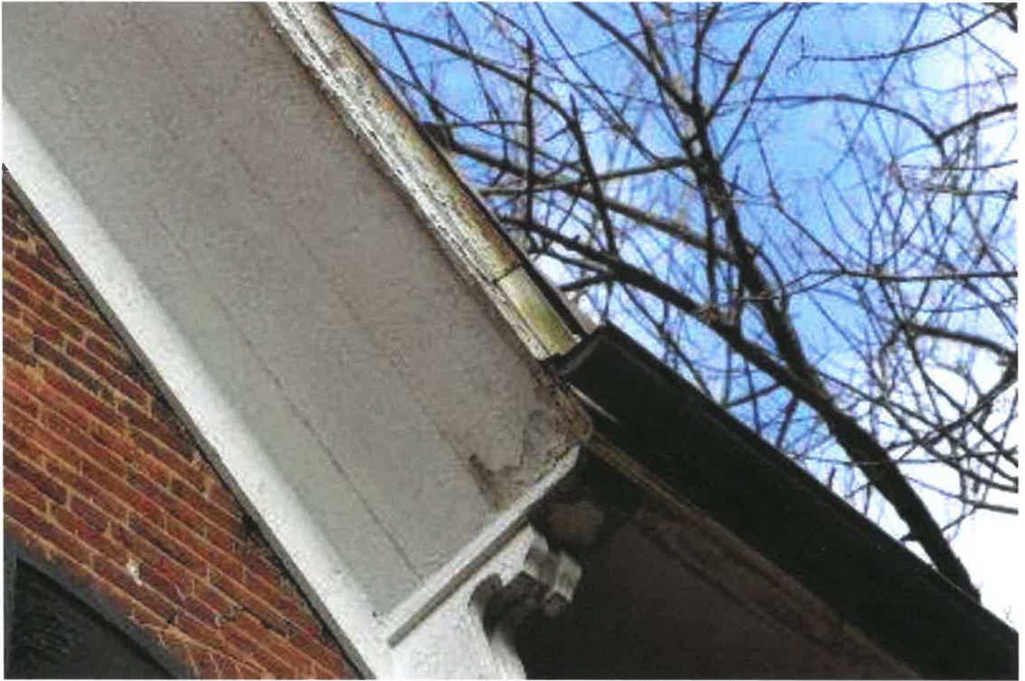
Roof Flashing and Trim Issues
