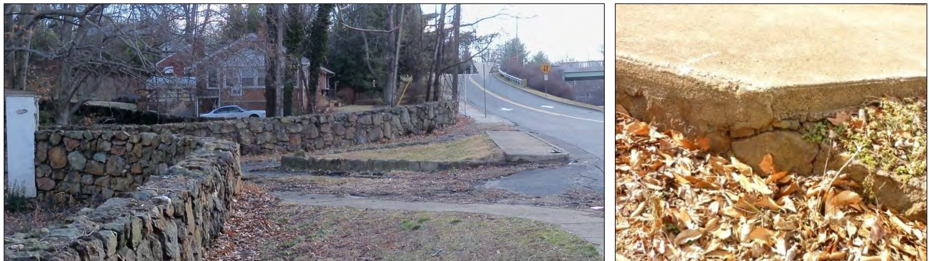
Photo 6: At Left, View of Historic Entrance and Parterre Looking East; at Right, Detail Juncture of Parterre and Sidewalk (Dovetail, February 2011).
