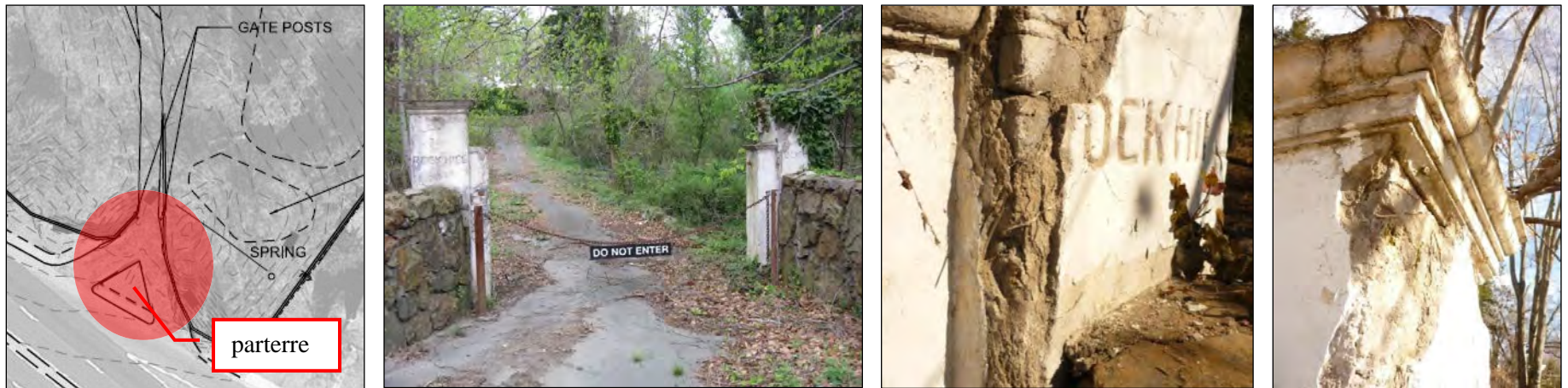
Photo 5: At left, South Elevation Historic Entrance Gateposts (C. Taniguchi, April 2010); at Center and Right, Details of Eastern Gatepost Deterioration (Dovetail, February 2011).
