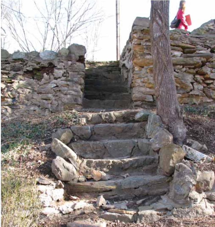
Deteriorating terrace 1 stairs and walls in February, 2011. Note the wall condition on the right.
