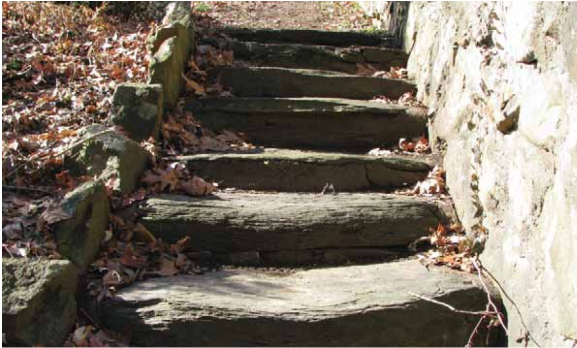
Stone stairway to woodland garden area. Note mortar deterioration (February 2011).
