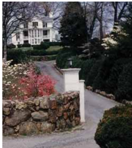
Left: East gatepost, 2011. Note damaged stucco, brick and concrete, with partially damaged inscription.
