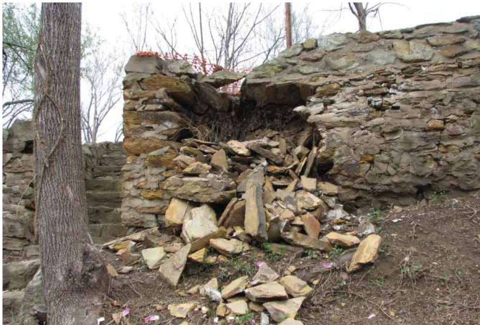
Failure of the same terrace 1 wall in March 2011.
