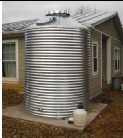
1500-gallon Rainwater Harvesting Systems for not-for-profit agency
