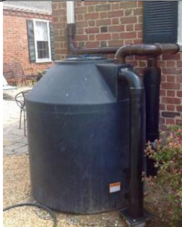
965-gallon Rainwater Harvesting System for residence
