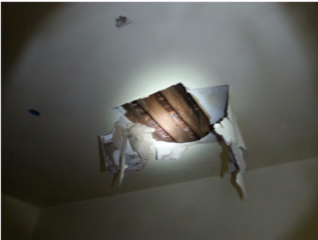
Photo 4 – Damaged ceiling area
