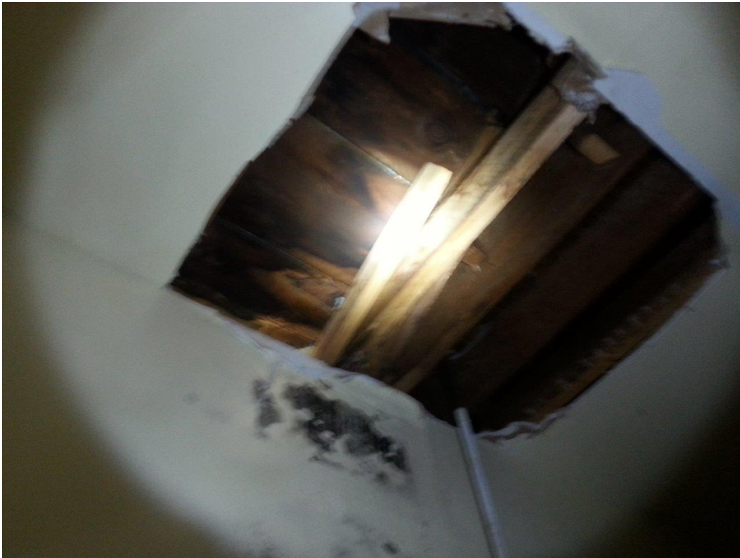
Photo 3 – Active leak, damaged ceiling, mold and deteriorated wood framing
