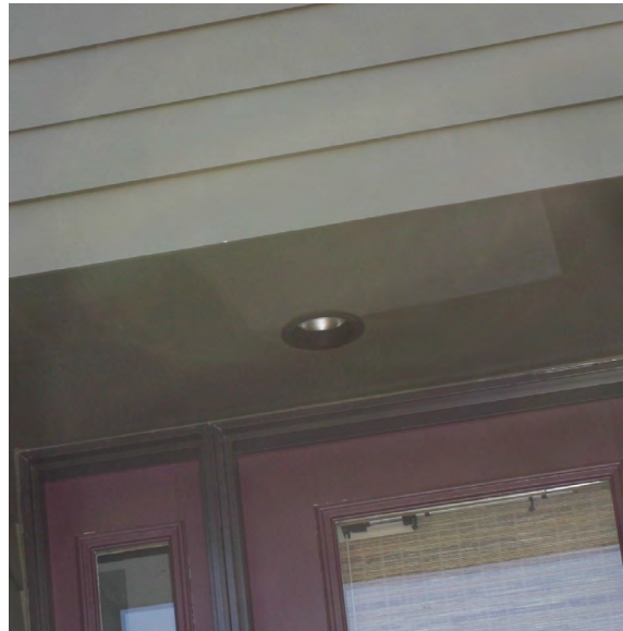
Recessed exterior soffit lights
