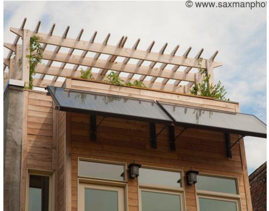
Building-integrated solar energy systems in residential districts
