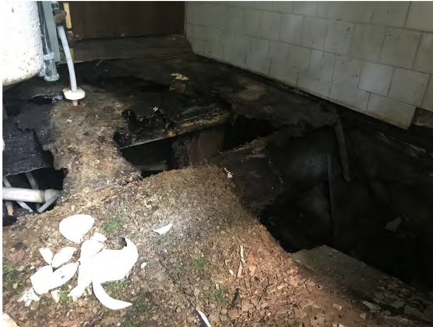
Interior detail – bathroom floor damage
