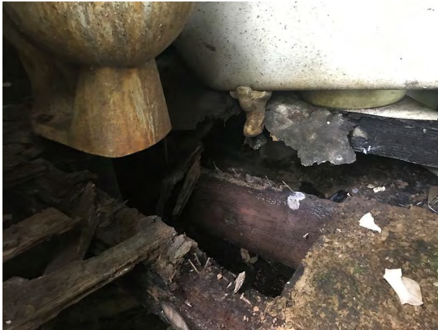
Interior detail – bathroom floor damage
