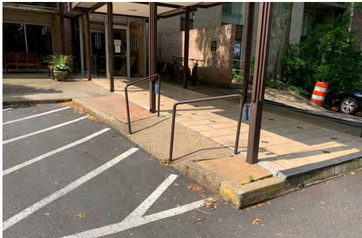
CURB RAMP IS NOT ADA-COMPLIANT
