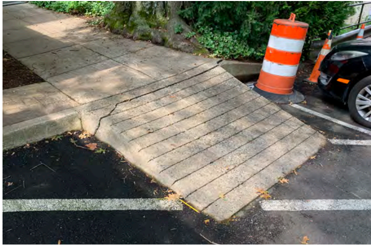
RAMP IS DANGEROUS TO NAVIGATE
