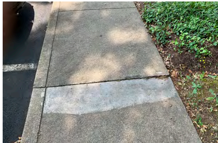
CHANGE IN LEVEL AT WALK JOINTS DOES NOT COMPLY WITH ADA REQUIREMENTS
