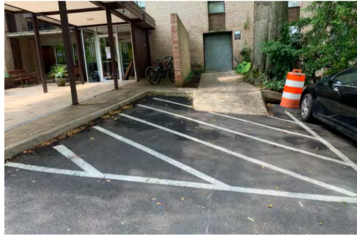
RAMP IS DANGEROUS TO NAVIGATE
