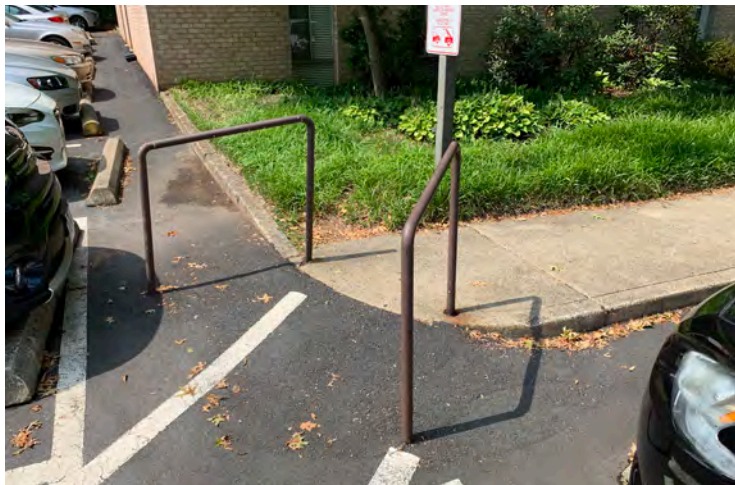
CURB RAMP IS NOT ADA-COMPLIANT
