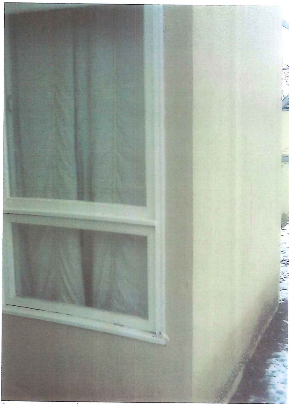
South-facing window to be replaced
