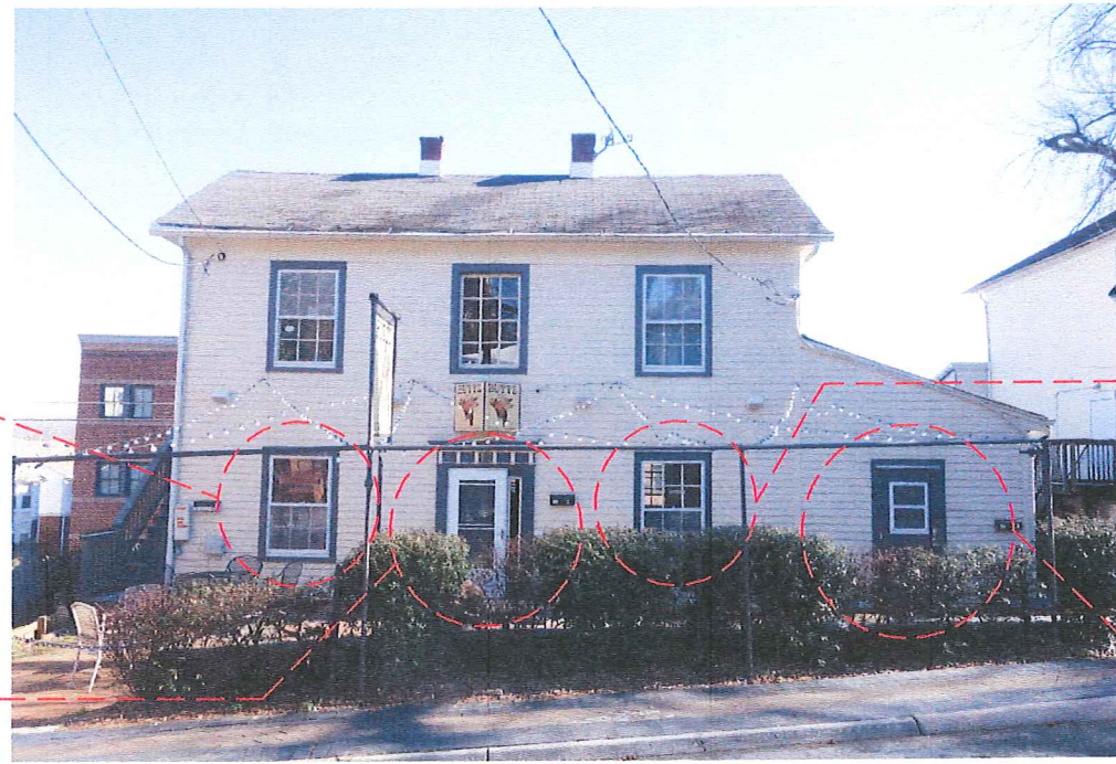
THE UPPER SASH OF THIS WINDOW IS NOT ORIGINAL TO THE BUILDING.
