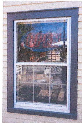
THE UPPER SASH OF THIS WINDOW IS NOT ORIGINAL TO THE BUILDING.
