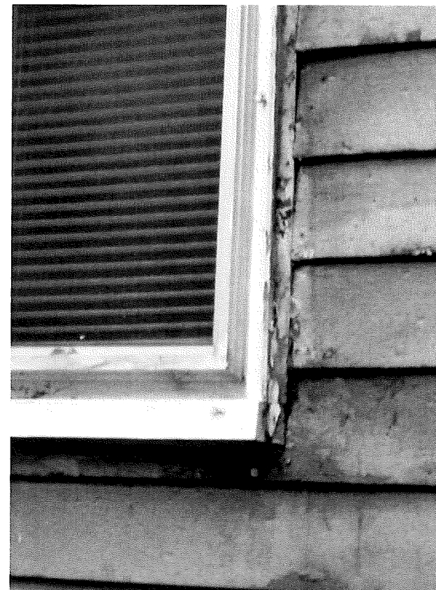
Condition of Existing Window Trim and Sill
