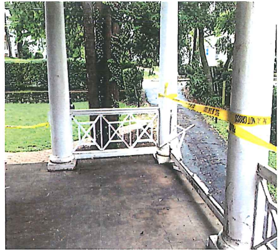
Broken Railing Area
