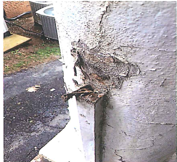
Missing Railing Connection
