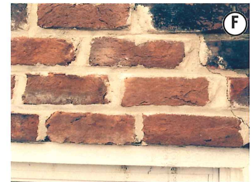
MASONRY IN POOR CONDITION
