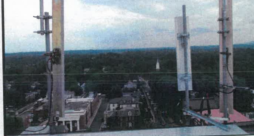
EXISTING ANTENNAS (NORTH)
