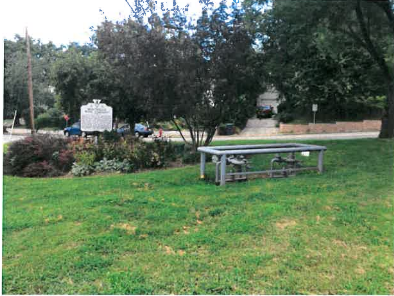
Gas regulations at McIntire and Perry Drive
