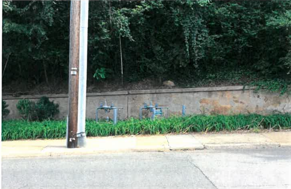
Gas regulation station on E. Market Street across from Vinegar Hill
