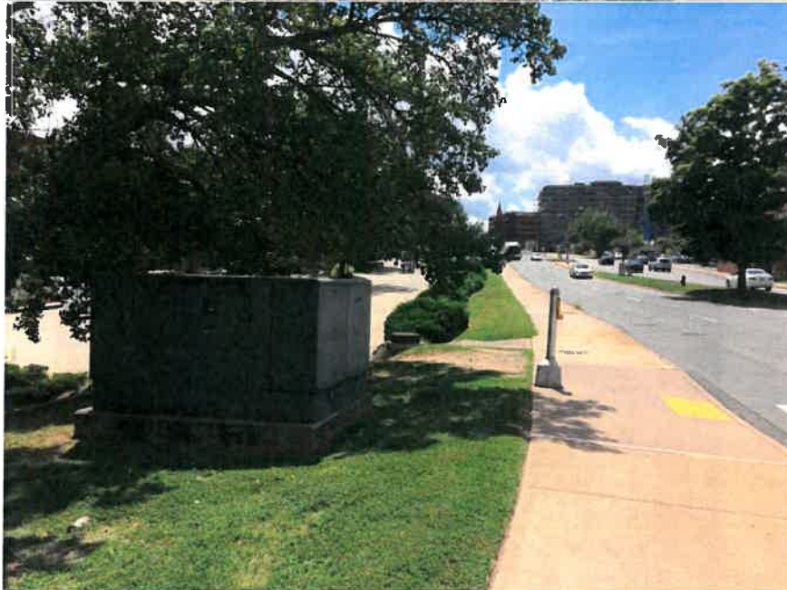
Power Transformers at Ridge/McIntire and Preston Avenue
