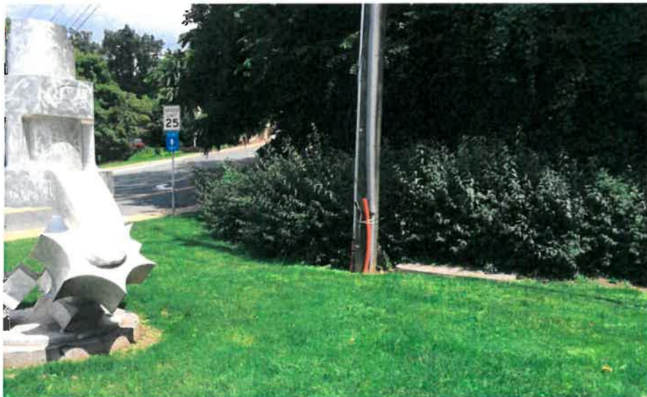
Above Grade Dominion Power vault hidden by vegetation.
