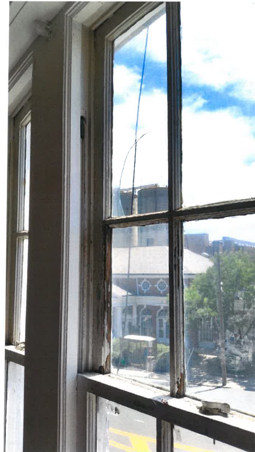
Sash cords are missing at most windows
