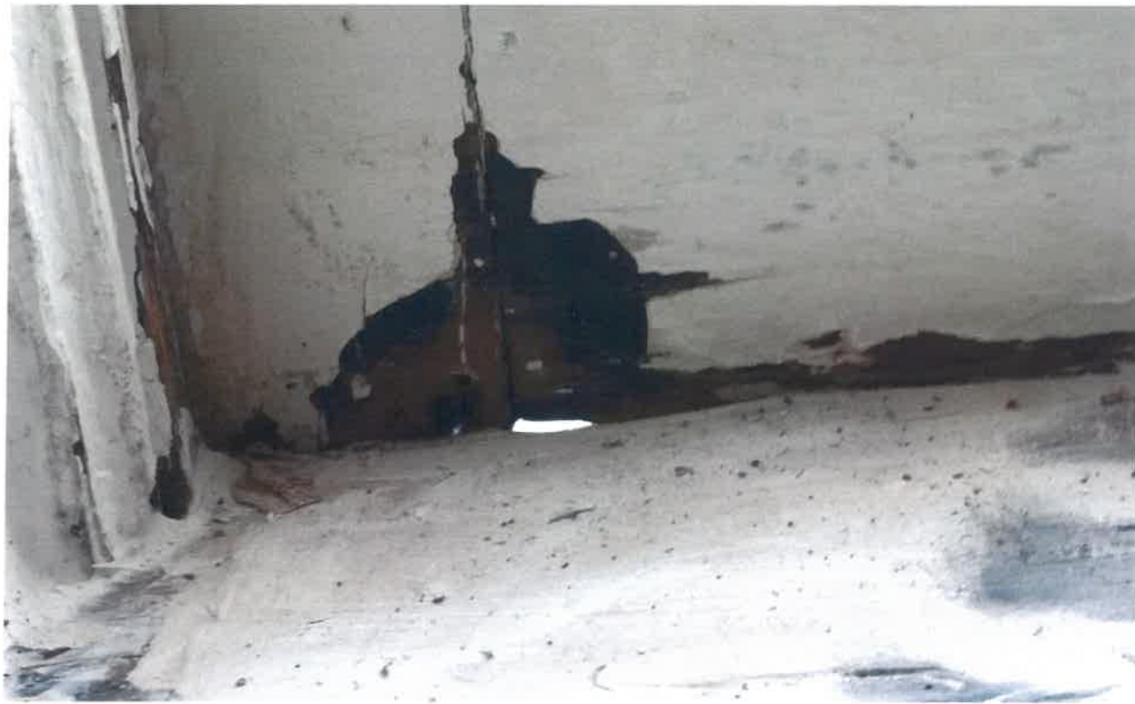
Poor condition of sash and stool.
