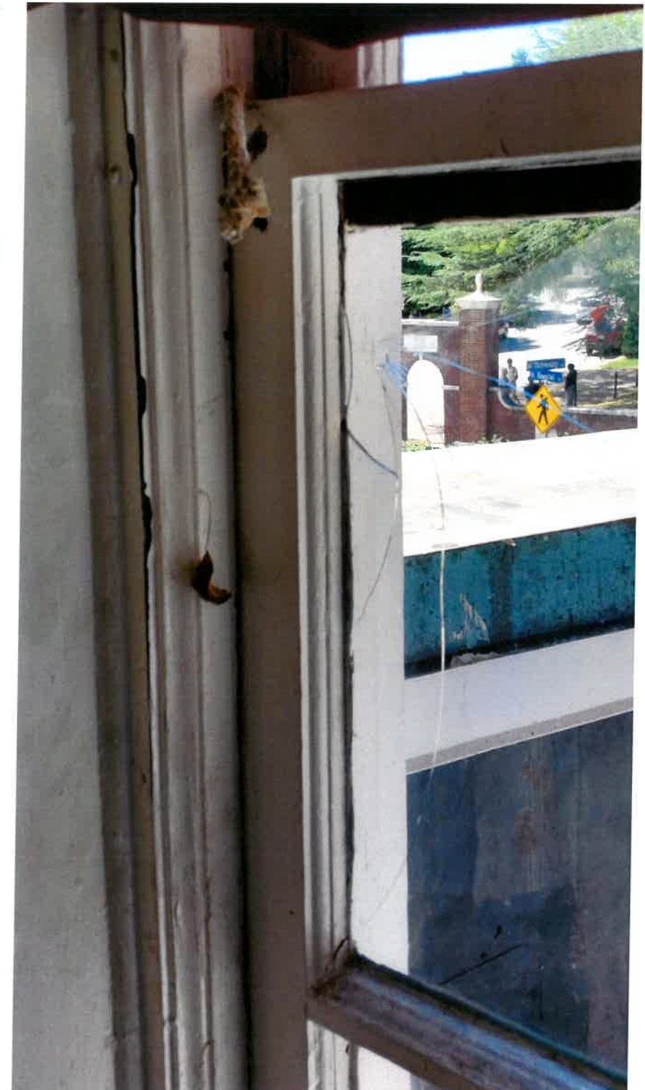
Many sashes are screwed together
