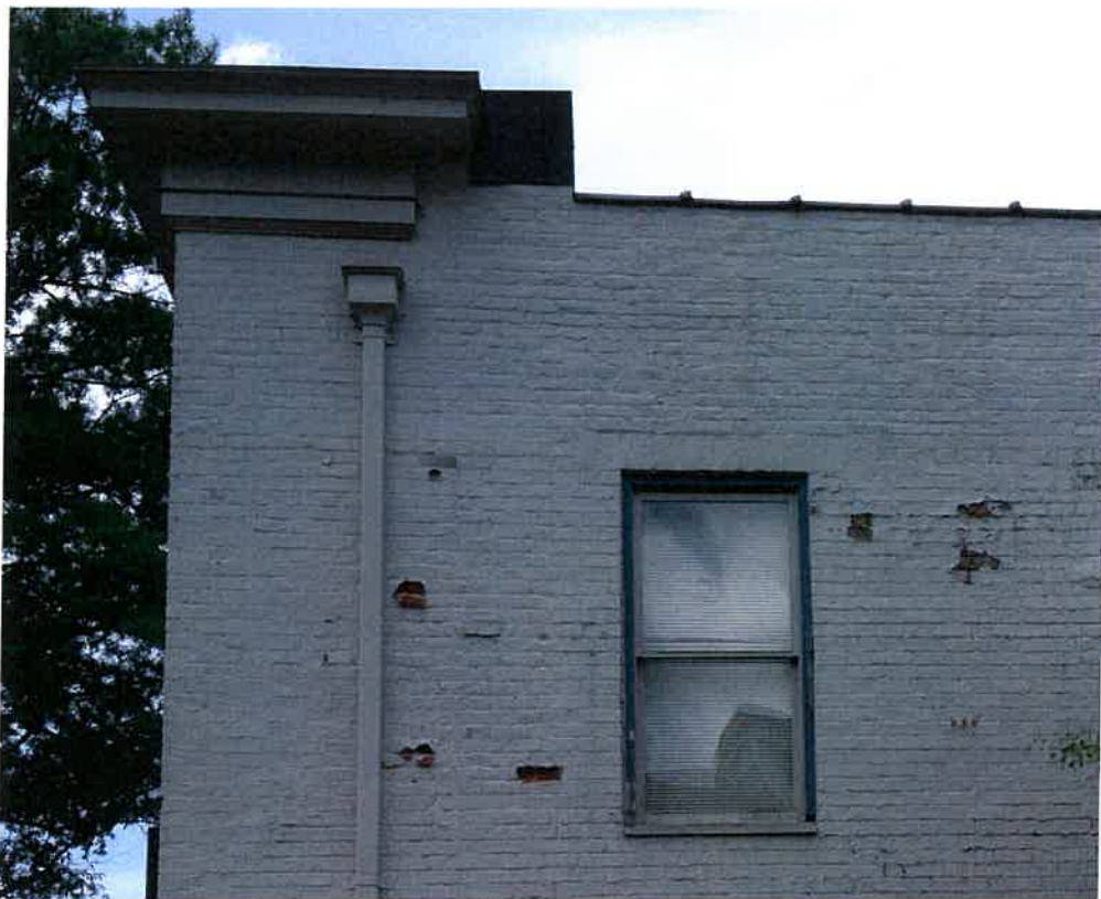
Photo of paint peeling and red brick beneath coating.
