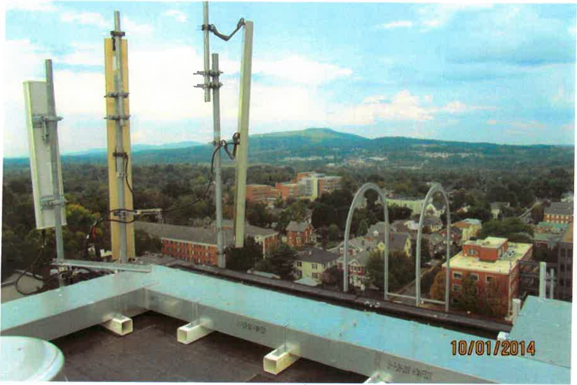
CV (101) (24) Ntelos antennas on penthouse To be removed
