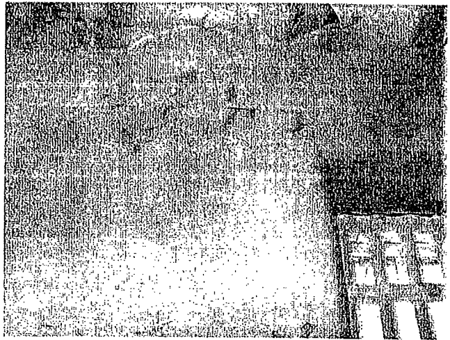
Settlement Crack in Granite Section
