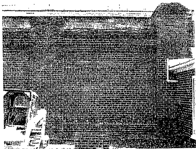
South Wall--Typical of Wall Condition (Note Lime Leachate Caused by Water Penetration from Top of Wall)
