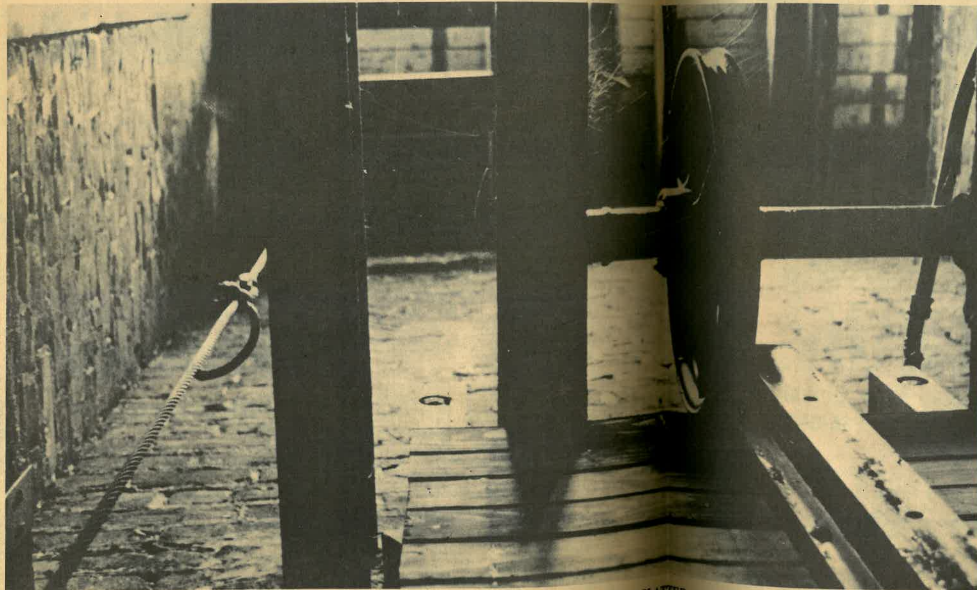
AN EMPTY ROOM STANDS BEHIND THE TOP OF THE NOW-UNUSED PINE-SLATTED OPEN FREIGHT ELEVATOR Investors Theorize That Renovation May Bring In 10 Medium-Sized Retail Stores
