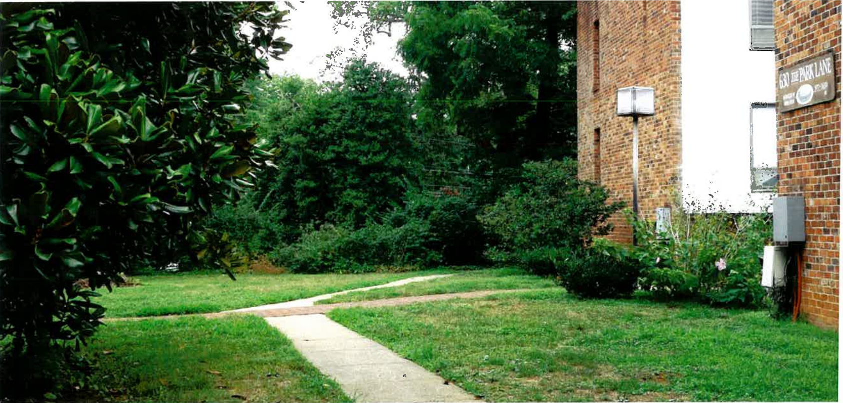
Existing concrete and curving brick paths to be removed. Light fixtures to remain.
