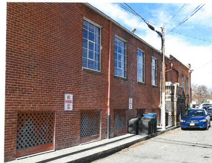
3 EAST ELEVATION LOOKING NORTH - EXISTING WINDOWS TO BE RESTORED WOOD STAIR AND DOOR TO BE REMOVED
