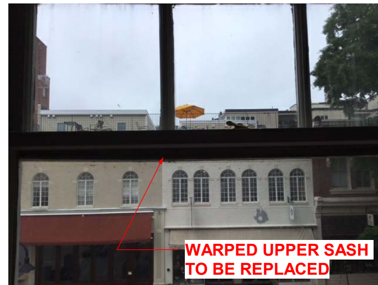
WARPED UPPER SASH TO BE REPLACED
