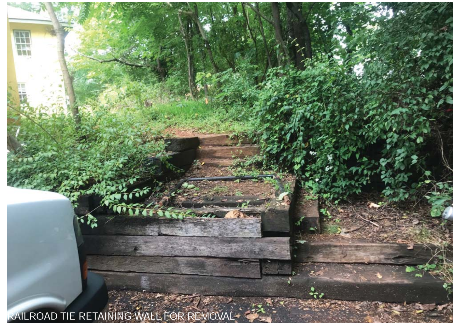
RAILROAD TIE RETAINING WALL FOR REMOVAL
