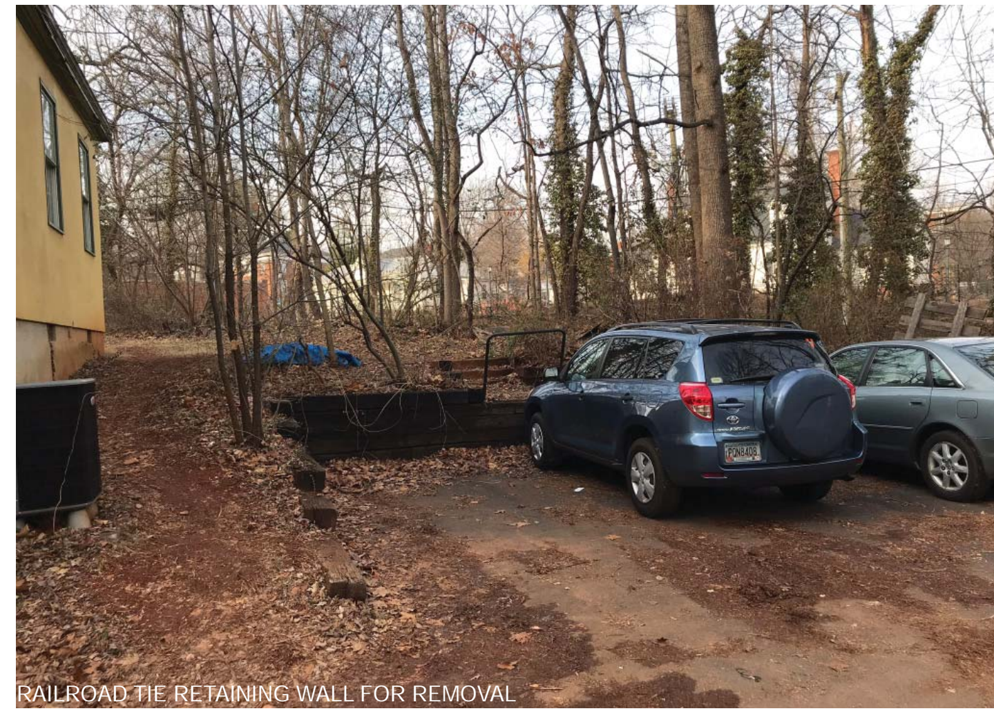
RAILROAD TIE RETAINING WALL FOR REMOVAL
