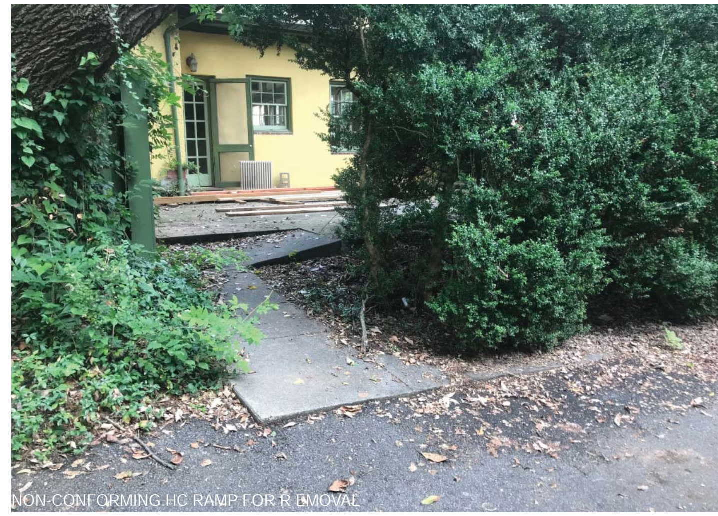
NON-CONFORMING HC RAMP FOR REMOVAL
