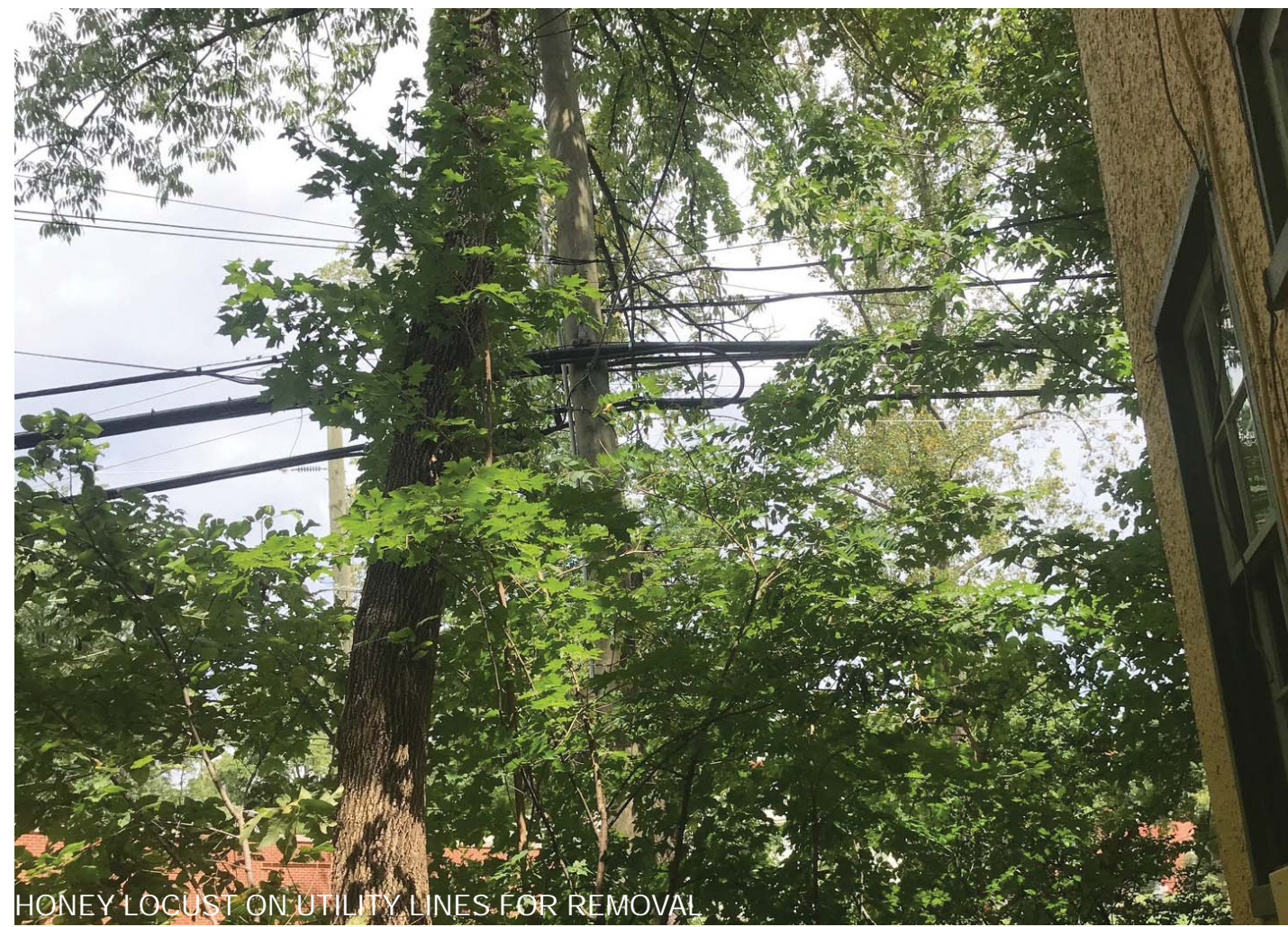
HONEY LOCUST ON UTILITY LINES FOR REMOVAL
