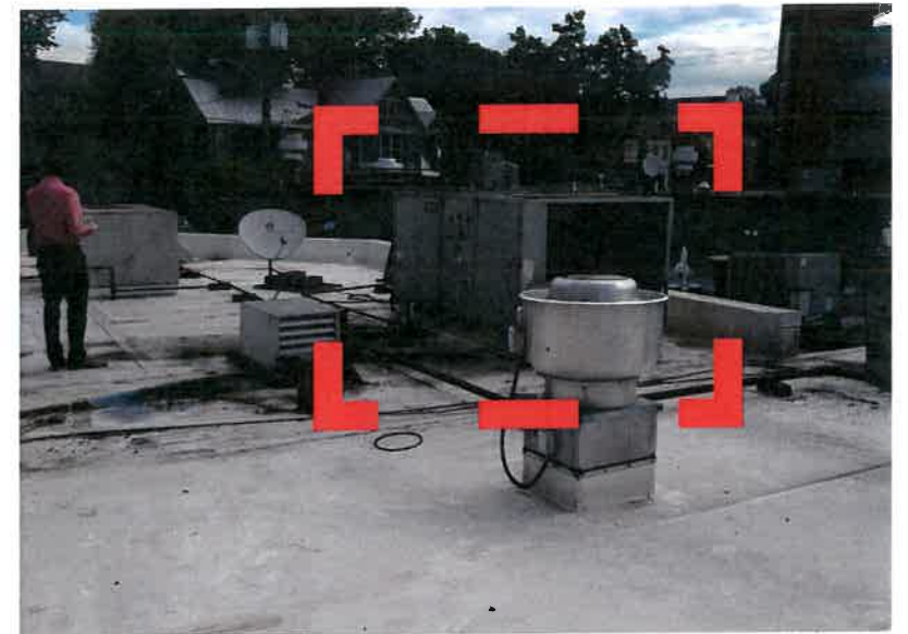
MECHANICAL UNIT TO BE REPLACED
