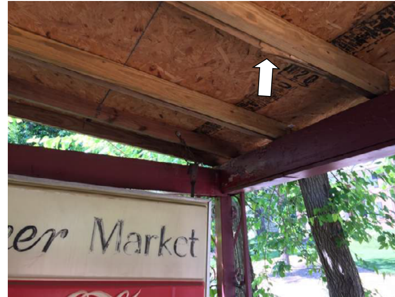
Undersized porch roof beams and rafters. Failed rafter at porch.
