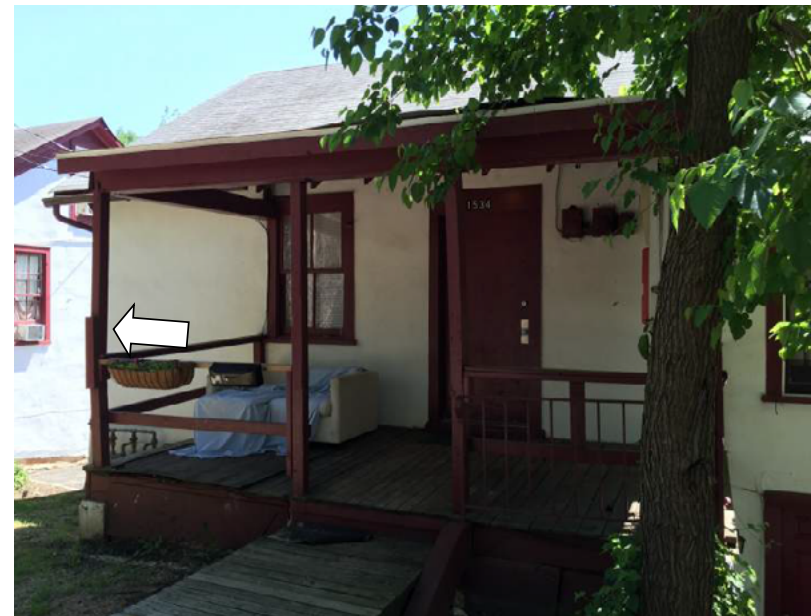
Corner post at porch is spliced and buckling.
