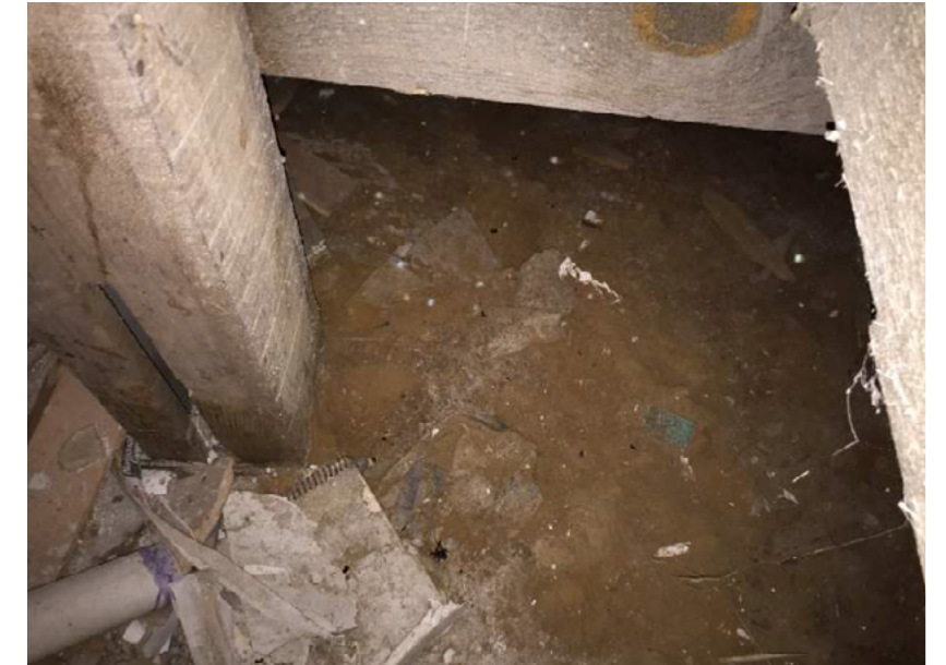
Low, damp crawl space with questionable foundation support for load
