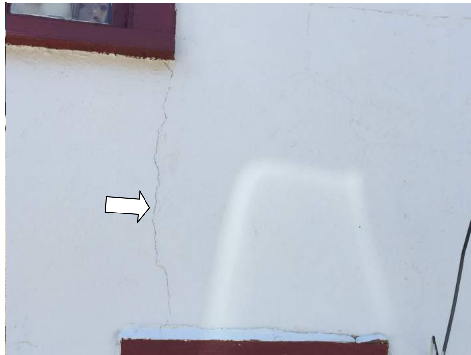
Cracking in exterior foundation walls
