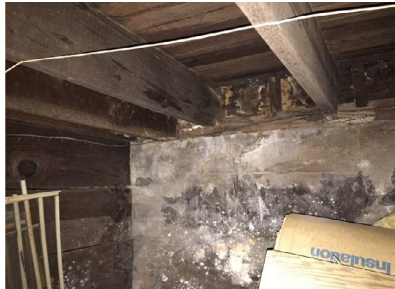
Water infiltration through foundation wall and damaged floor framing.
