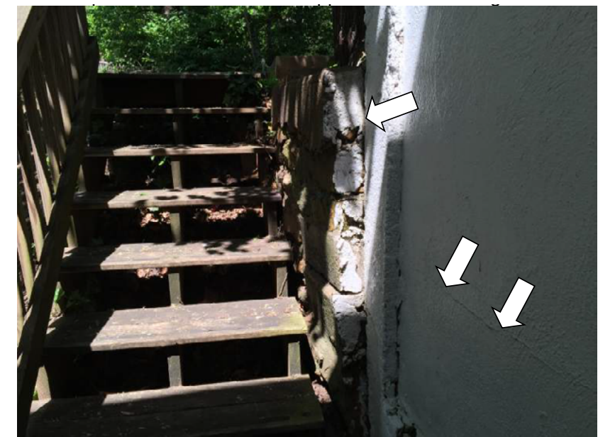
Cracked foundation wall and leaning stacked masonry retaining wall.
