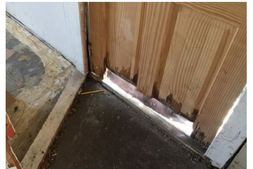
Water infiltrating lower level floor.
