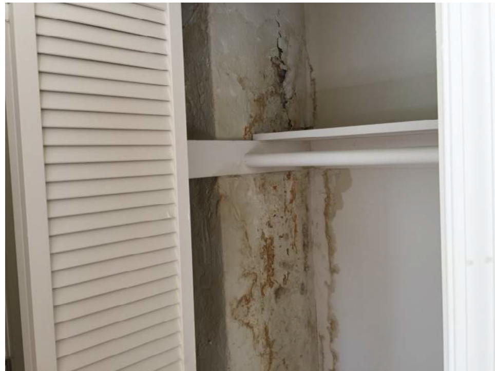
Water infiltration through old chimney.
