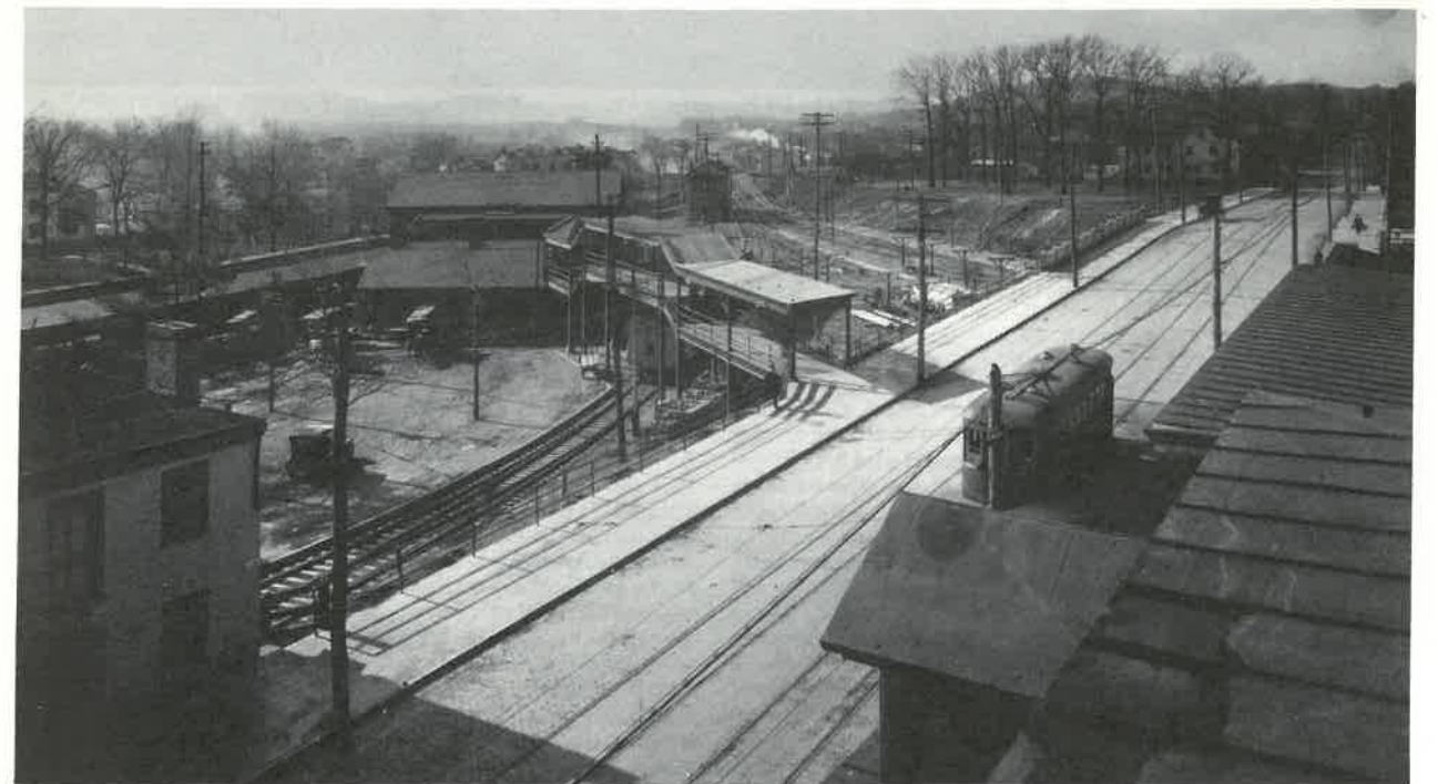
Top: Car 21 uses temporary track eastbound while track is laid on the new overpass over the Southern Ry. The Hotel Clermont is at the right. 8 May 1918. Holsinger.
