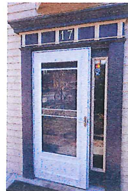
THE ENTRY DOOR AND SIDELITE ARE NOT ORIGINAL
