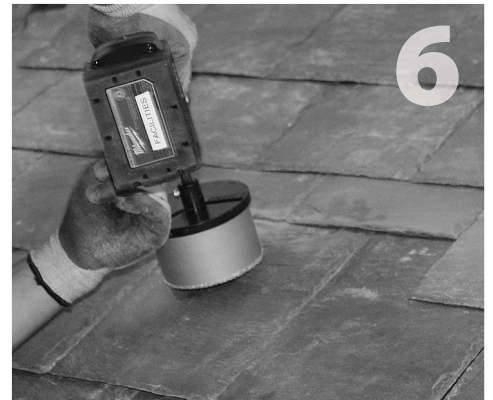
Using a 4" diameter diamond hole saw and the pilot hole drilled in step 3, drill through the existing slate.
