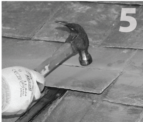
To remove the slate below the score, slightly lift the lower portion of slate with a slate ripper, then gently but firmly tap the top piece with a hammer. The lower piece should break off cleanly.
