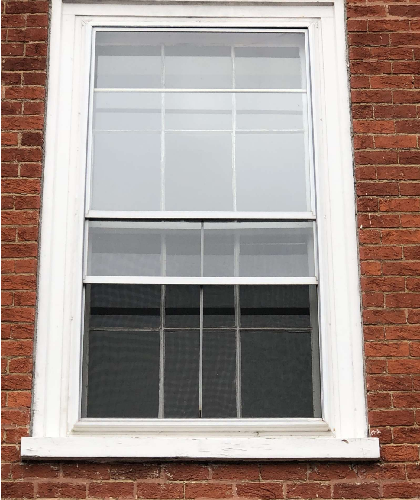
PHOTOS 1 -4 ORIGINAL WINDOW – NOTE MORTAR AT EDGES
