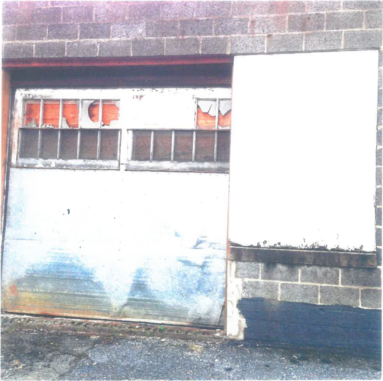
Existing sliding service door showing Condition no. 1
