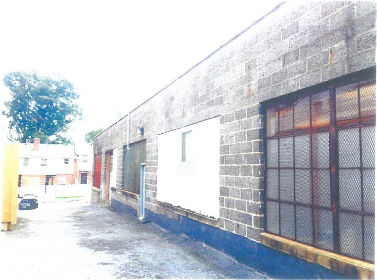
Remaining portion of north façade showing Condition no. 2
