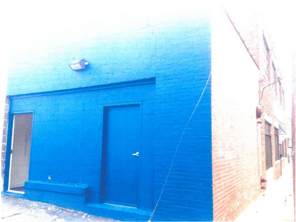
Northwest corner showing Condition no. 3
