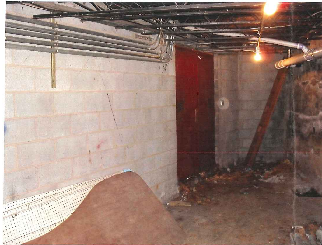
EXISTING DOOR ENTRY WALL - DOOR TO BE REMOVED AND NEW OPENING TO BE ADDED CMU TO BE STUCCOED; CONDUIT COVERED; BAR JOISTS EXPOSED
