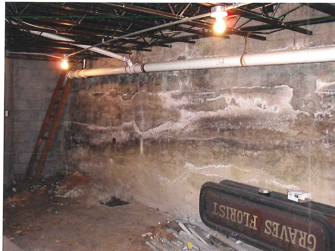
EXISTING INTERIOR WALL - SECTION OF WALL TO BE EXPOSED TO THE EXTERIOR
