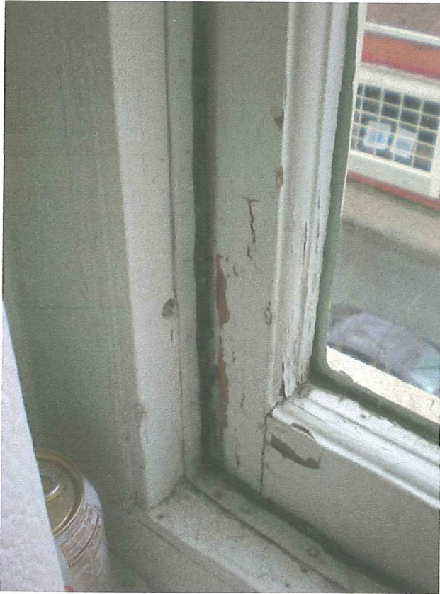
Applied metal trim @ damaged wood sash
