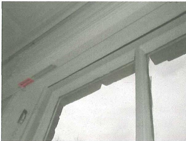
Upper sash not aligned in frame
