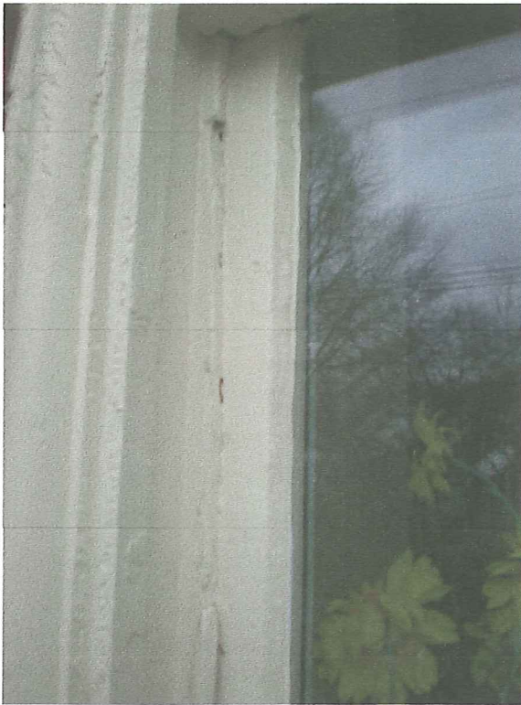
Damaged exterior stop
