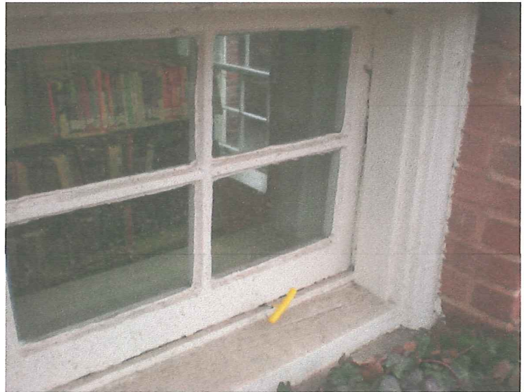
Casement window not tight to stops
