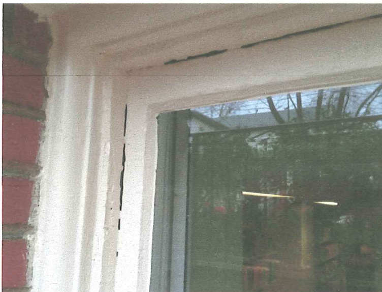
Gaps at exterior sashes
