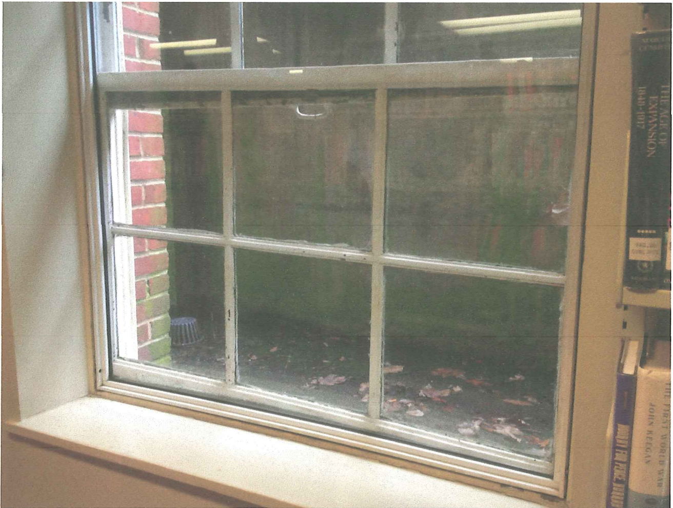
Misaligned bottom sash at metal window - basement NE corner
