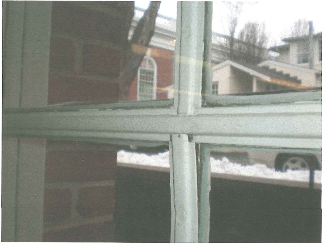
Examples of damage to metal frame and sash windows at north facade
