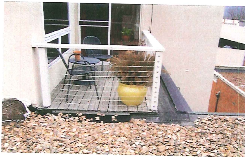
Replacement of wood decking is not included in our budget. Demolition is included since it will be necessary to do so for roof replacement.
