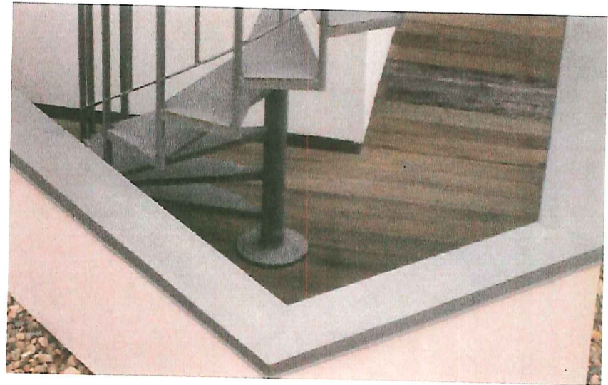
This stair will need to be removed along with the decking in order for us to properly re-roof underneath. Removal and replacement is not included.
