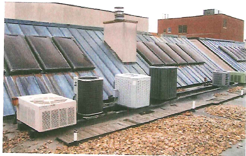
The sleeper rails that support the heat pumps need to be removed and replaced in a new position that doesn't block water from the copper roofs.
