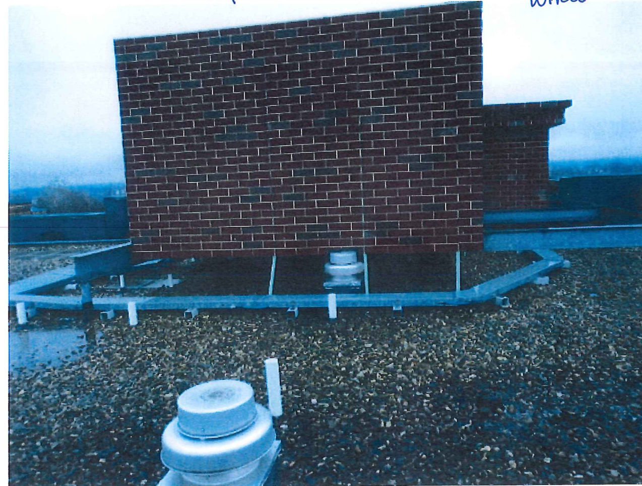
AT&T ENCLOSURE, EXISTING CABINETS BEHIND WALLS
