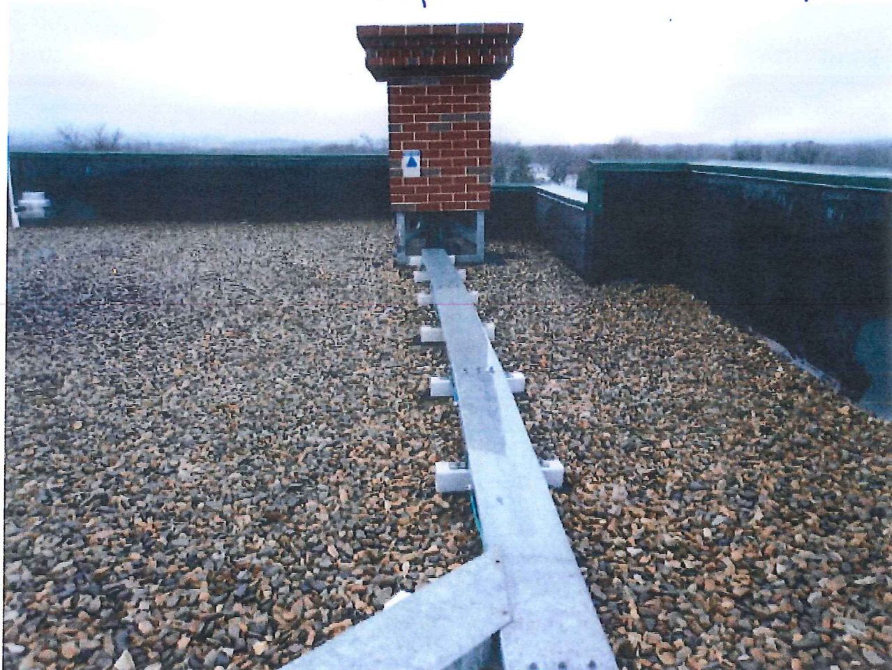
AT&T ENCLOSURE FOR EXISTING ANTENNA
