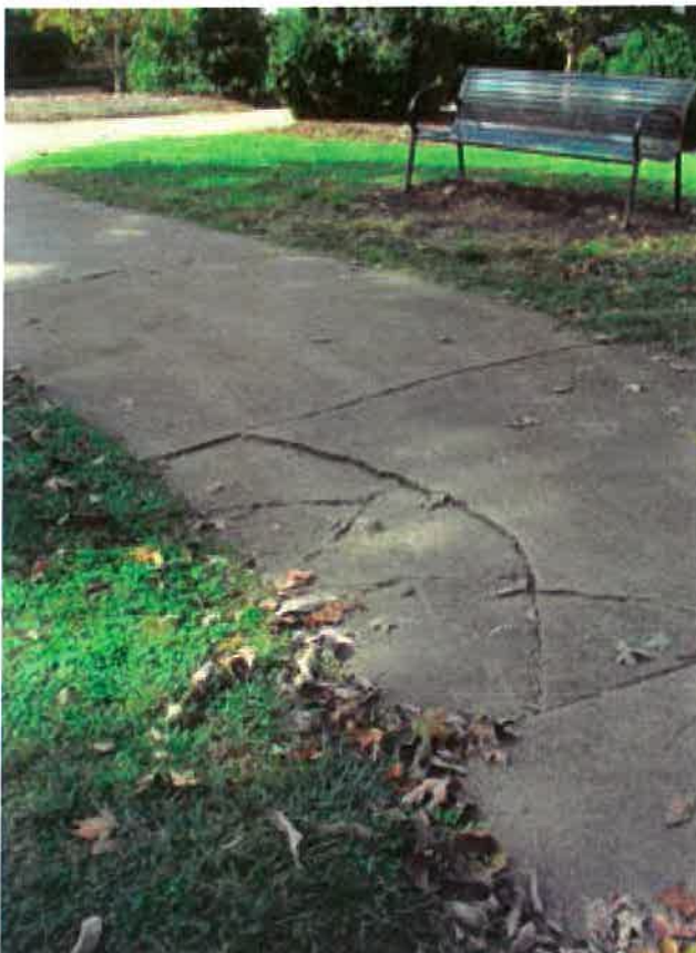
Photograph 19 - Typical Concrete Sidewalk Damage
