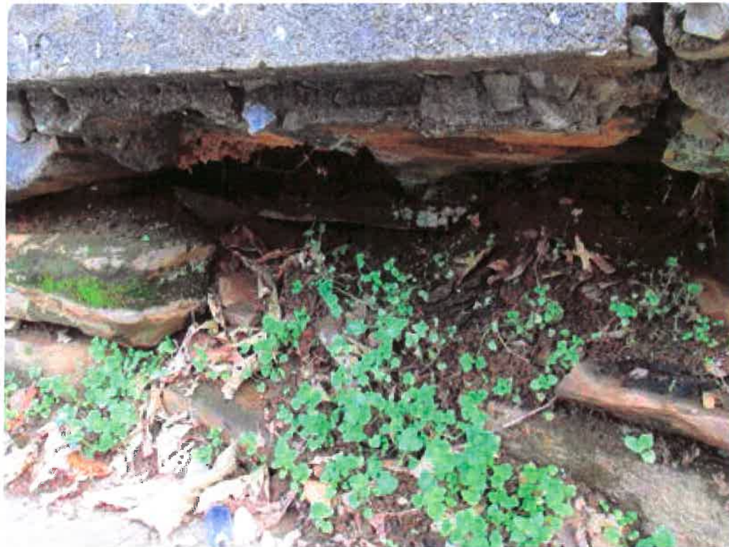
Photograph 12 - Erosion of Retained Earth
