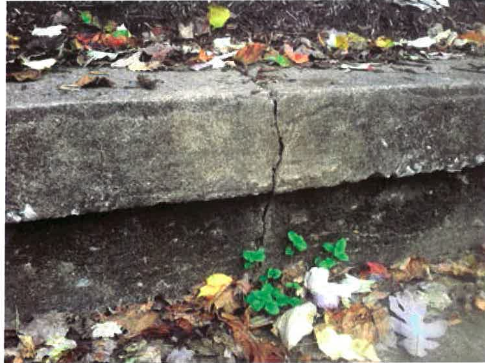
Photograph 19 - Transverse Crack in Concrete Retaining Wall
