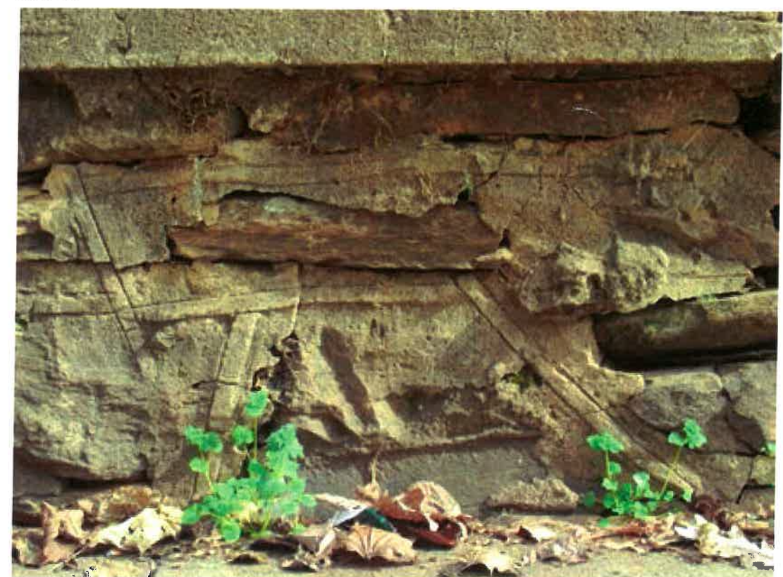
Photograph 5 - Remaining Parge Coating Along West Elevation
