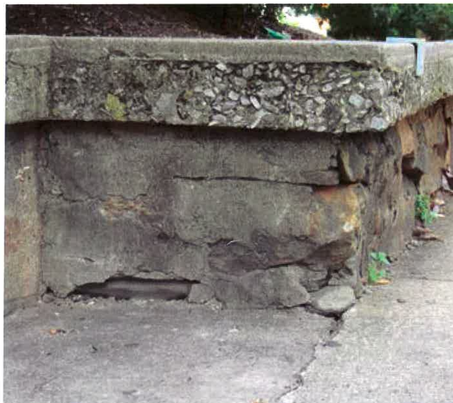
Photograph 14 - Concrete Cap Revealing Exposed Aggregate
