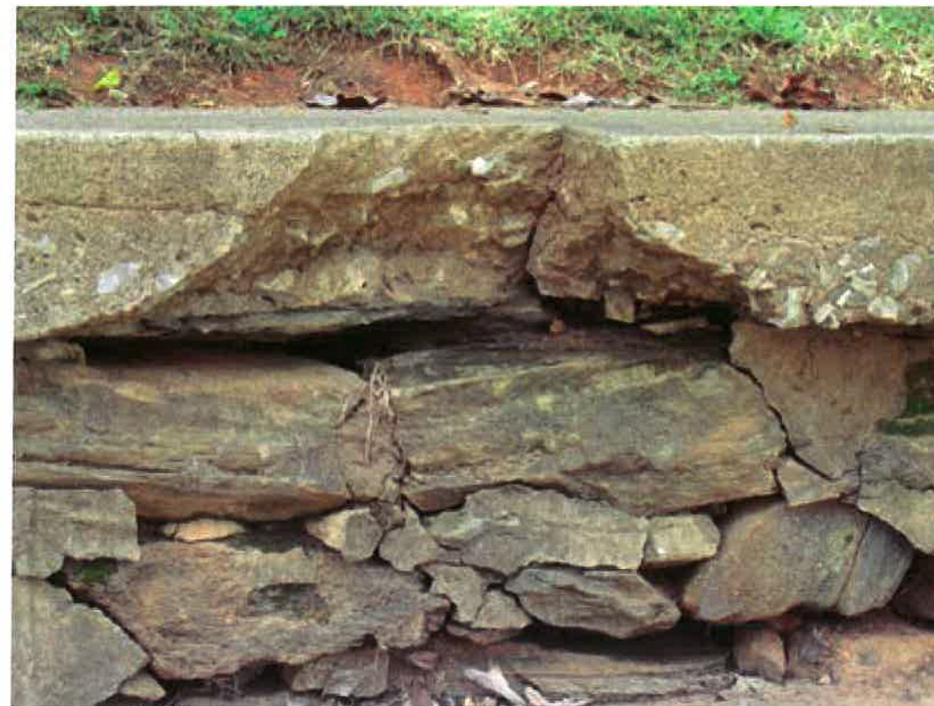
Photograph 15 - Damaged Concrete Cap (Note Absence of Reinforcement)
