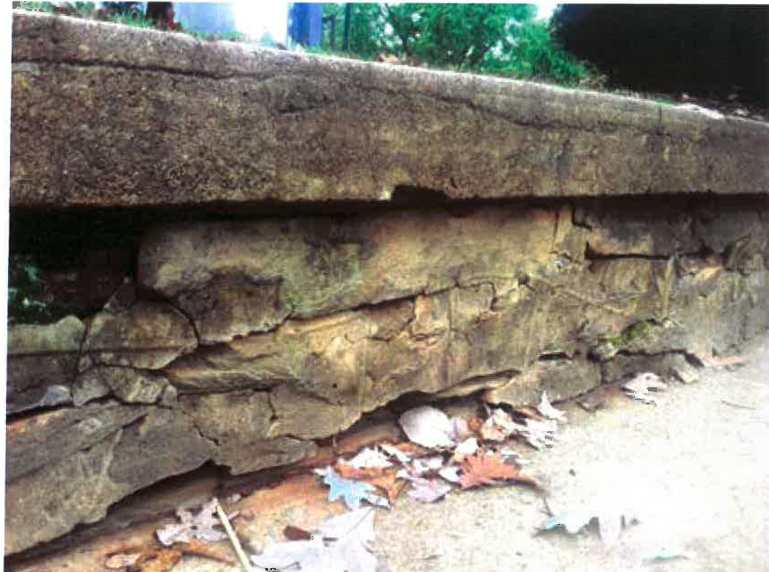
Photograph 2 - Remaining Parge Coating Along East Elevation (note raised read tooling marks)
