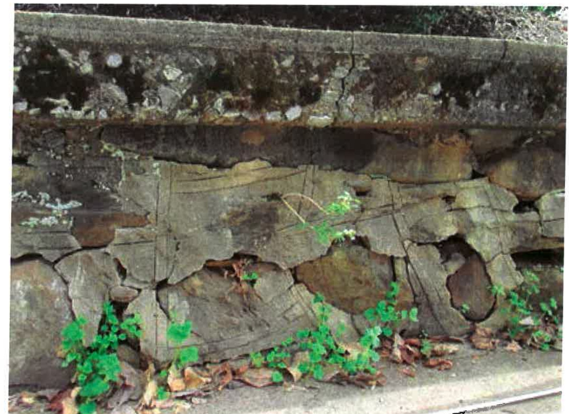
Photograph 3 - Remaining Parge Coating Along West Elevation (note double struck tooling marks)
