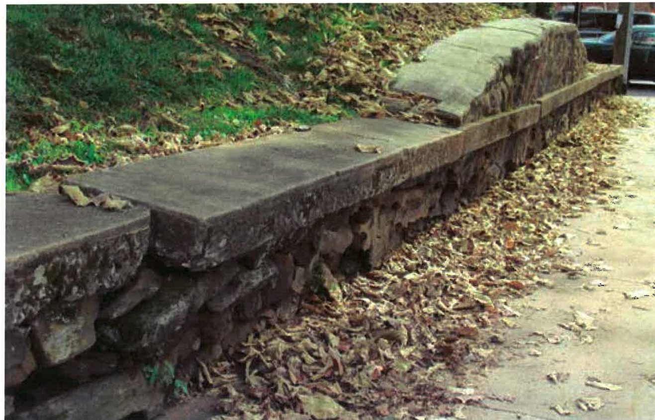
Photograph 11 - Existing Wall Showing Concrete Cap Dislocation
