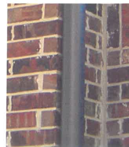
RAINWATER LEADERS - 4-INCH COPPER
