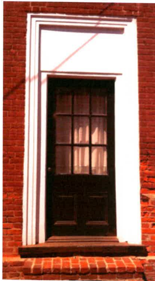
Example of door in a larger opening (perhaps a window.) Court Square.
