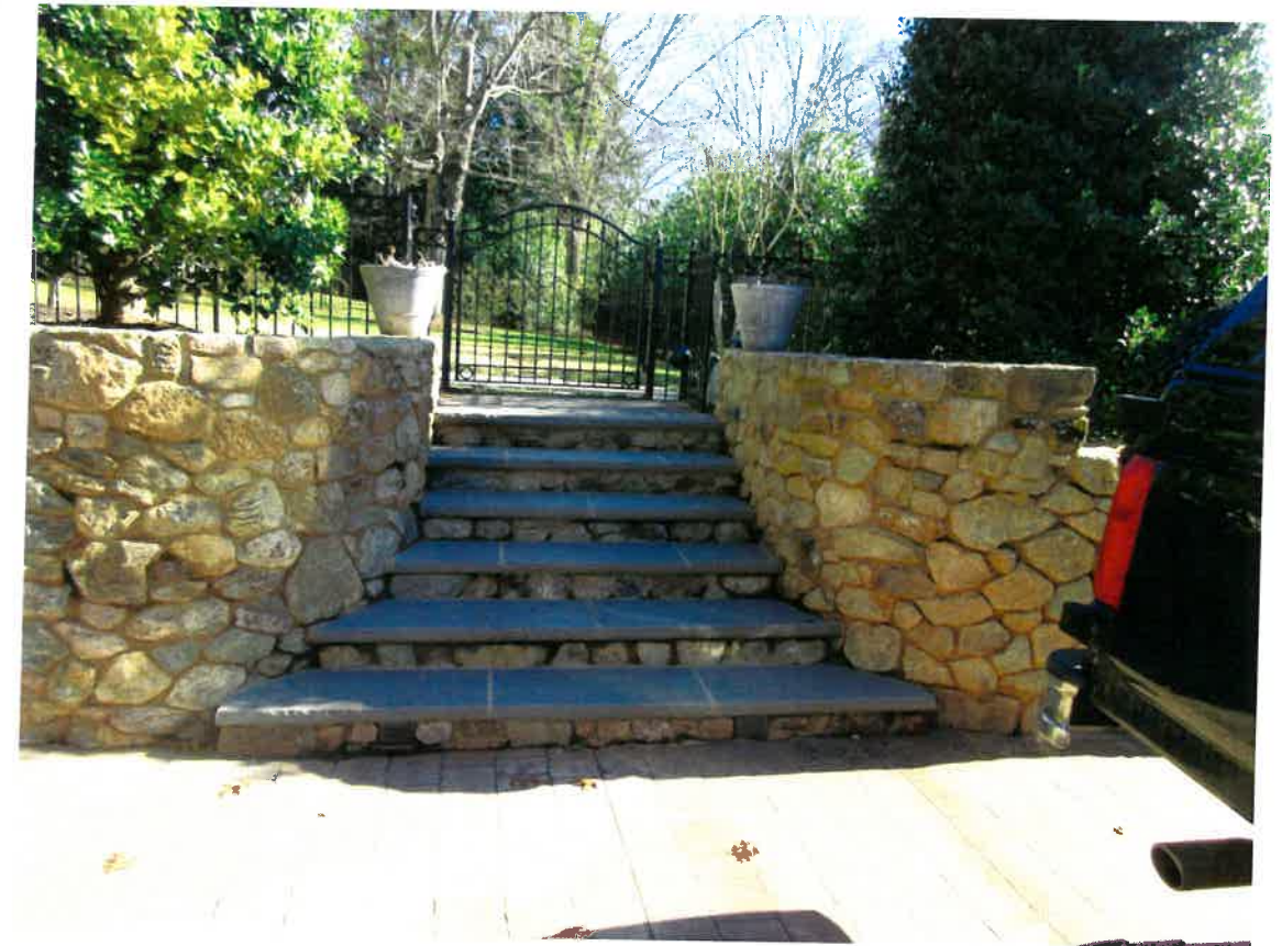
The new walls, concrete apron and walkways will match existing materials on-site.
