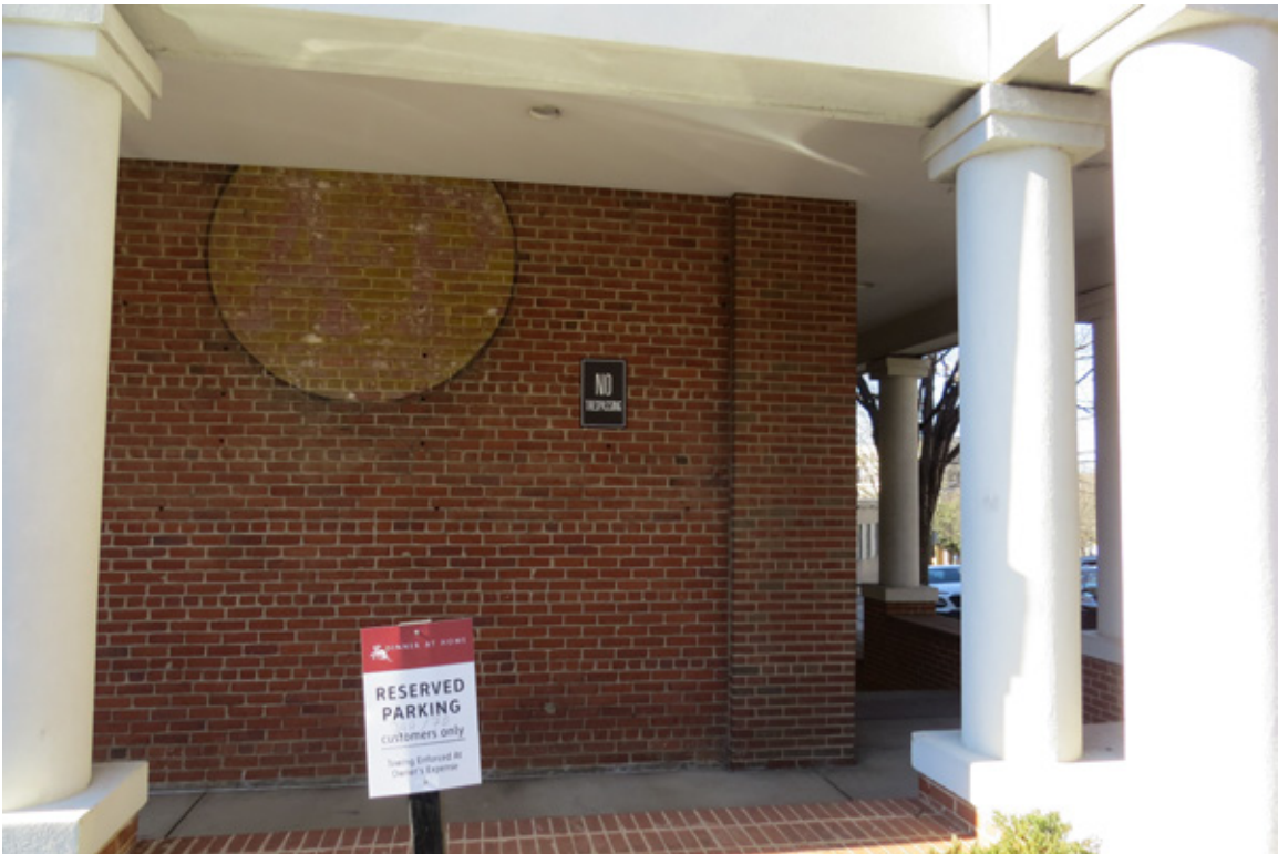
Northeast corner of the building: brickwork from three different periods of construction
