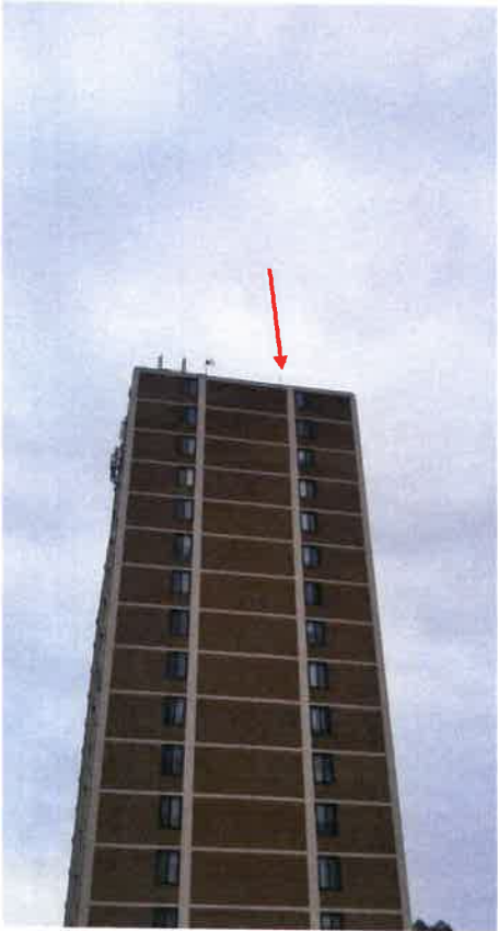
Pipes not concealed
