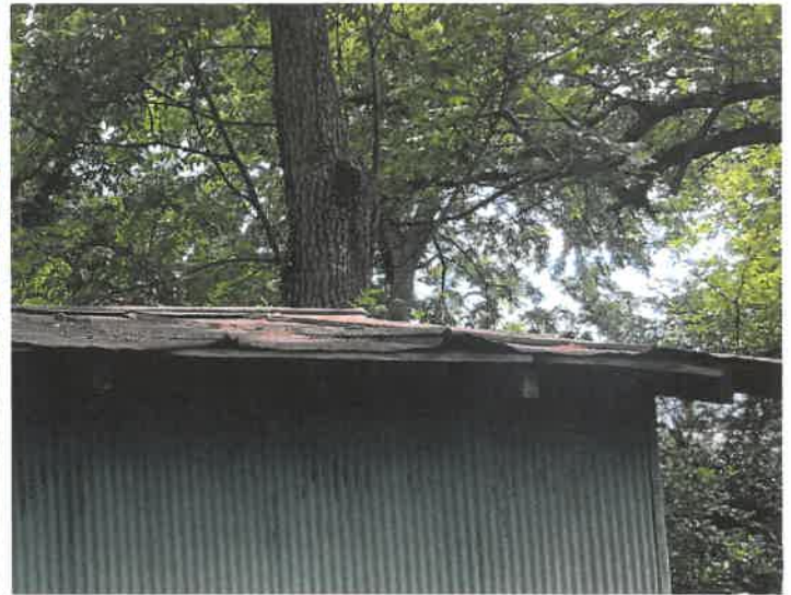
Damaged sheet metal roofing
