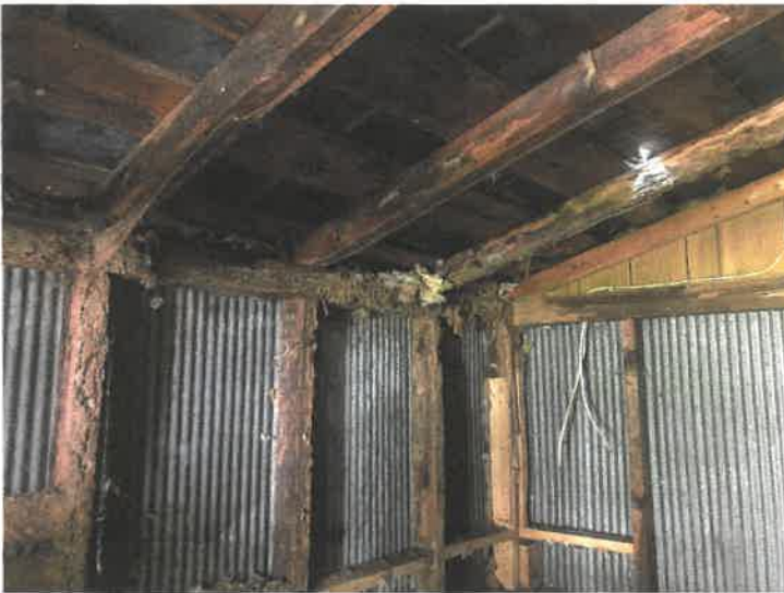
Holes visible through roofing
