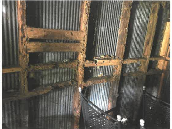
Rotting in original stud wall framing
