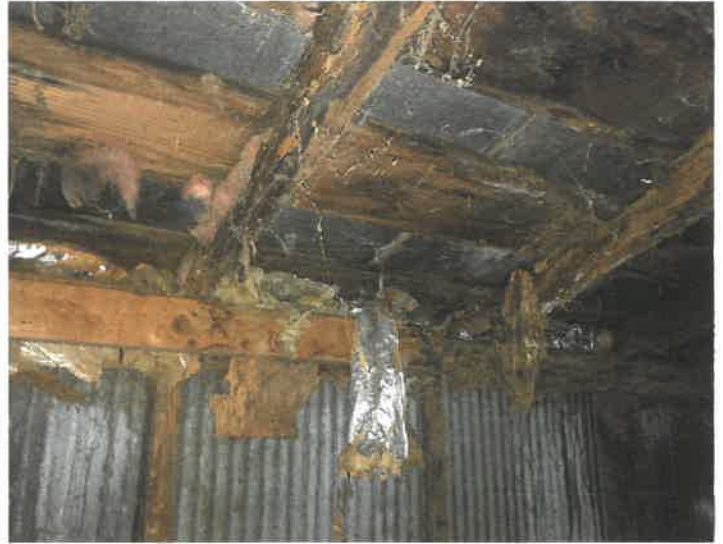
Substantial rot in existing wood framing
