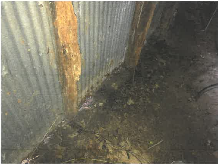
Rotting/water infiltration along north facade
