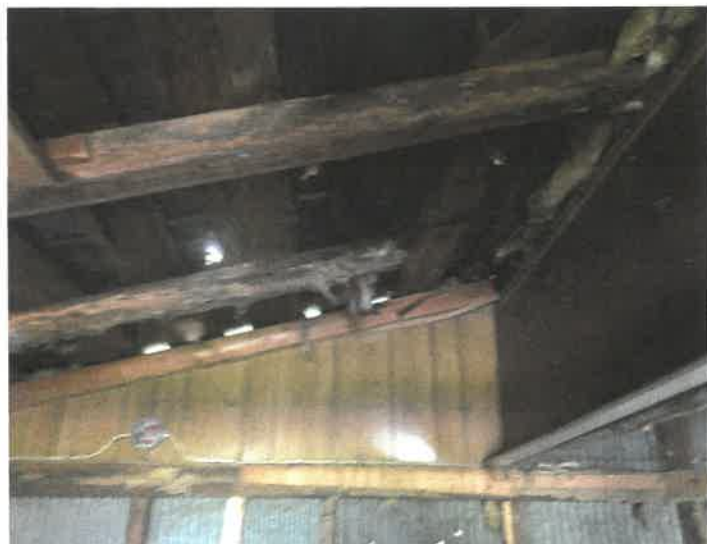
Rotted Roof Rafters
