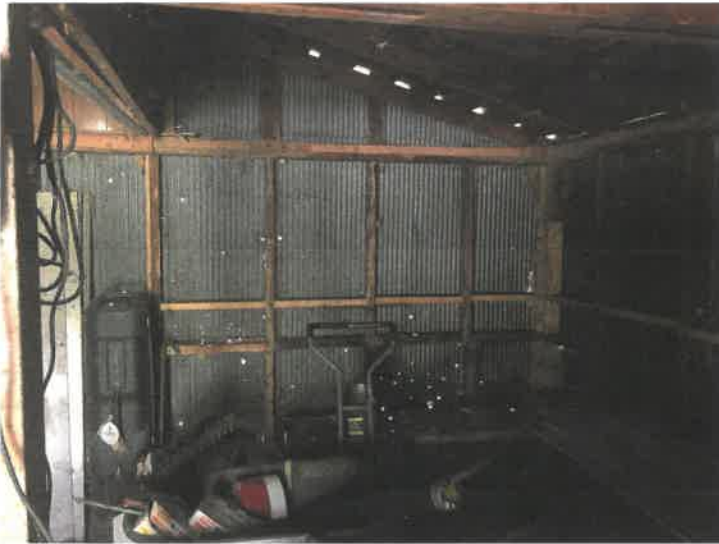
Numerous bullet holes and various penetrations
