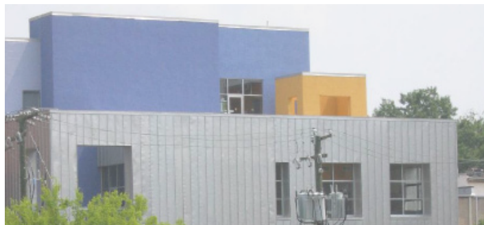
In commercial areas, the only location available for the placement of utilities may be the roof of the building. In this case, care should be taken to screen mechanical systems from view, as seen in this example.
