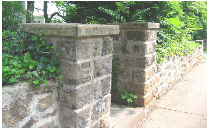
A low stone wall accented with evergreen plantings provides a historically appropriate border between a private lot and the sidewalk.
