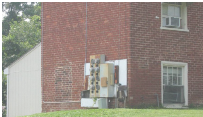
Strategically placed plantings would screen the view of this utility area from passerbys in this residential neighborhood.
