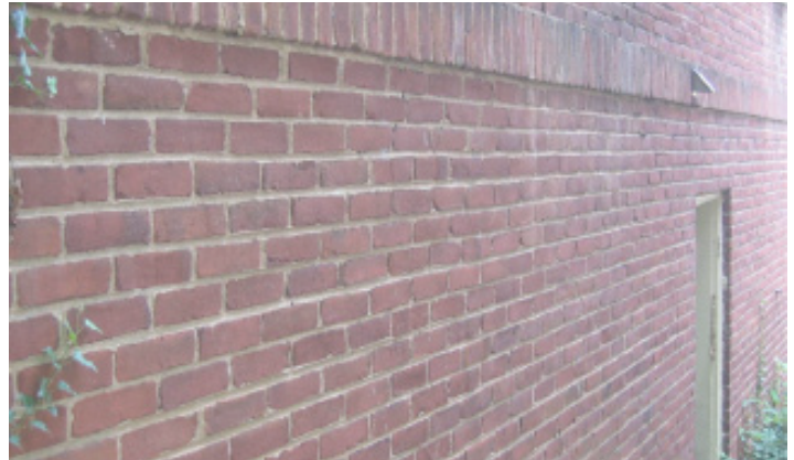
A running bond foundation is capped with a soldier course water table.
