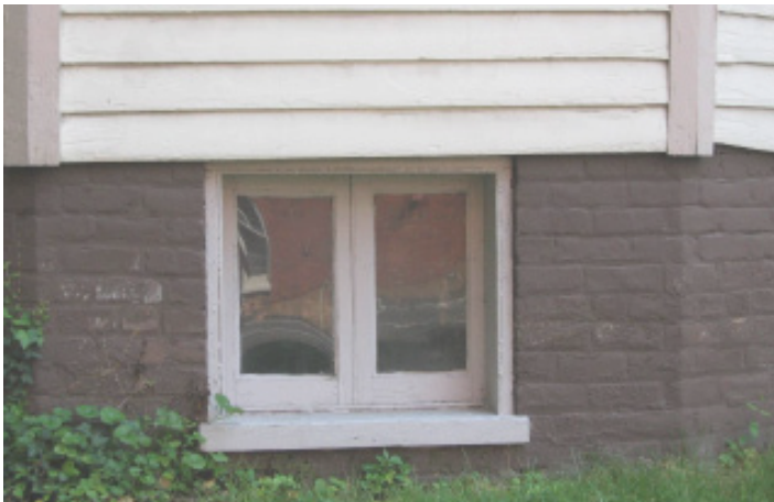
Brick laid in a running bond pattern are commonly used for residential foundations in Charlottesville.
