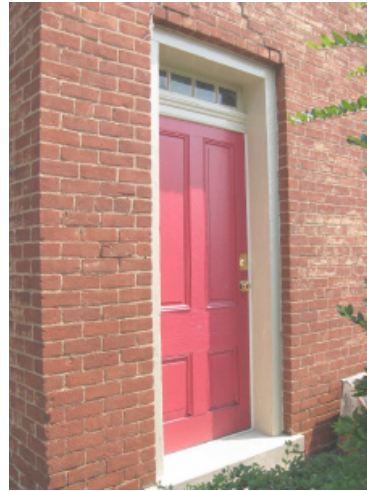
A raised panel door with transom above is a common feature of Federal and Colonial Revival architecture.
