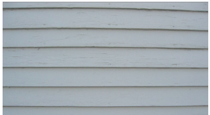
Horizontal boards that are flat or beveled are referred to as weatherboard and are common to a wide variety of architectural styles.
