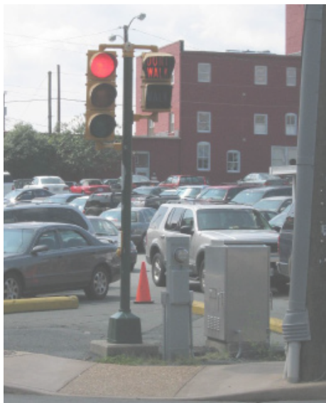
Situated next to a pedestrian-scaled traffic signal, control boxes are difficult to screen.
