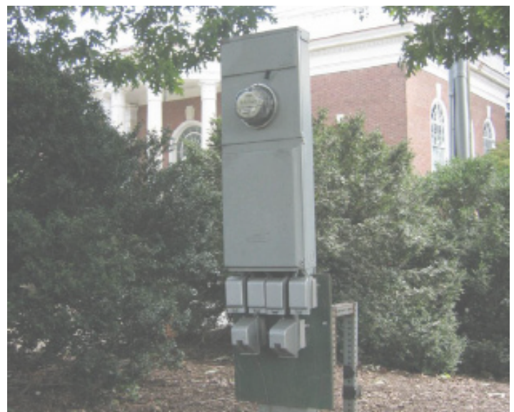
Service connections for the park are well screened from the adjacent street and surrounded by plantings while allowing access as needed.
